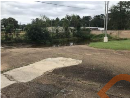
Northeast site drainage problem
