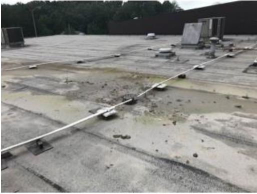
Failing modified bitumen roofing
