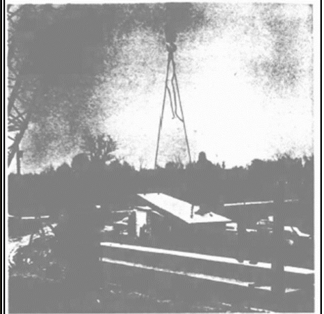
It's a free ride for a workman as the crane picks one of the huge beams up from the truck-trailer it arrived on, swings it buildingward.
