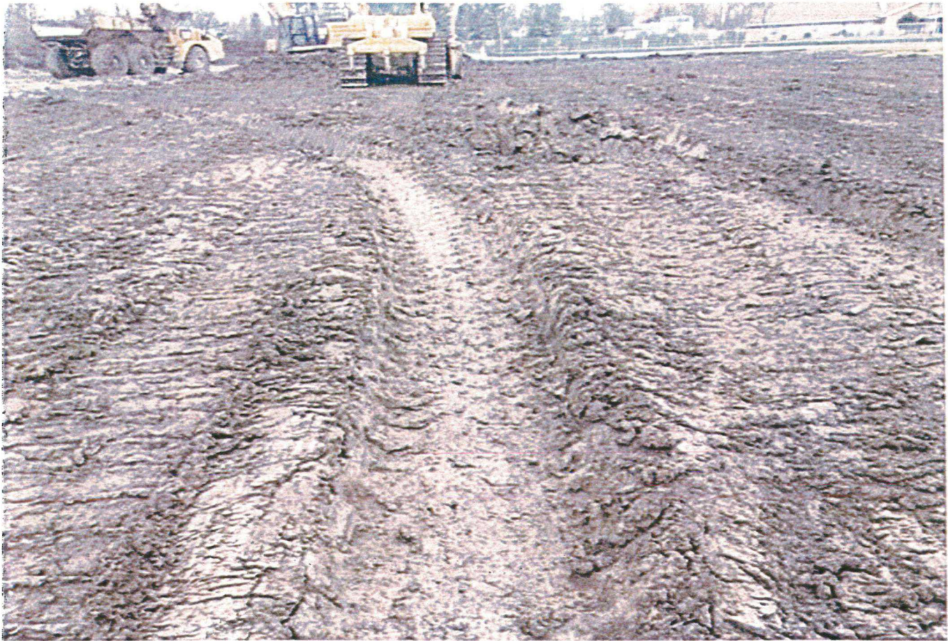
View of rutting of soils following proof roll.
