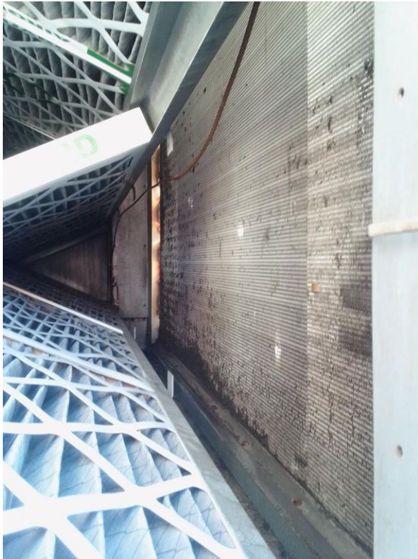
RTU-01 Heating Coils
