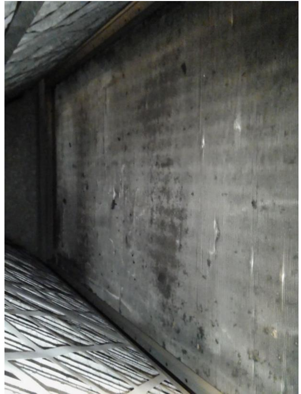
AHU-06 Heating Coils
