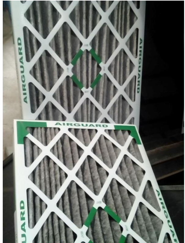
AHU-15 Mixed Main Filter Cleanliness
