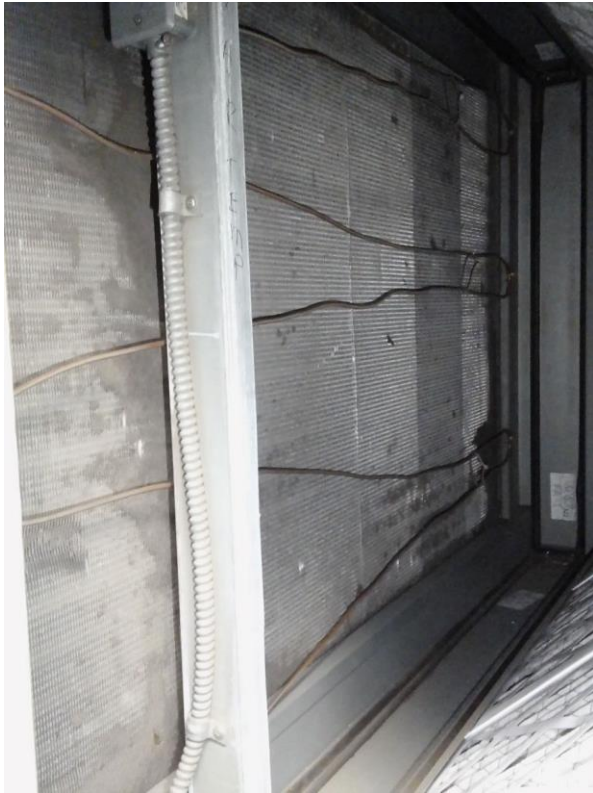
AHU-14 Heating Coils
