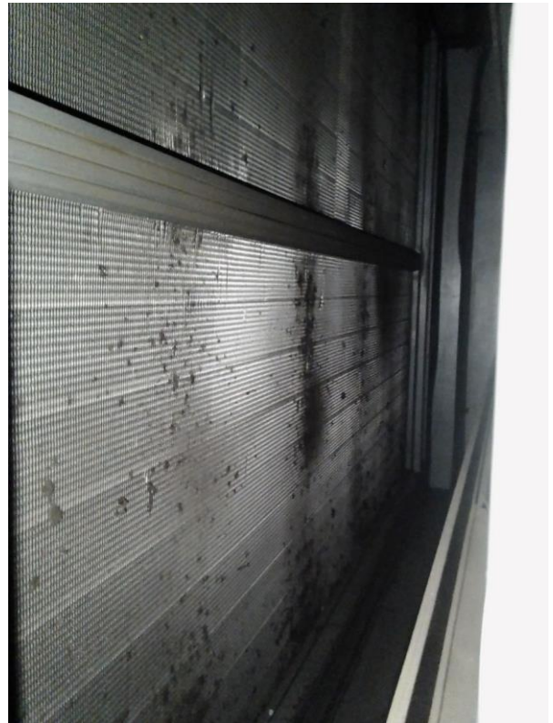
AHU-08 Heating Coils
