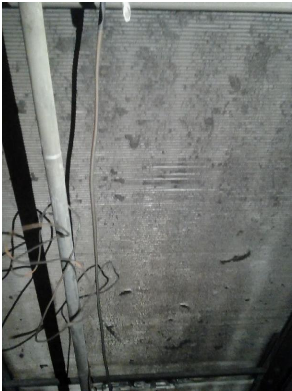
AHU-15 Heating Coils
