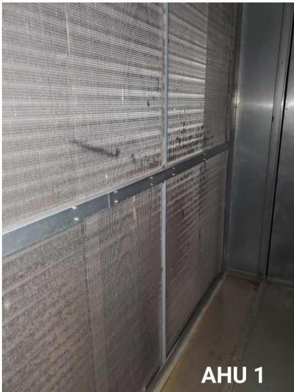
AHU_01 Cooling Coils
