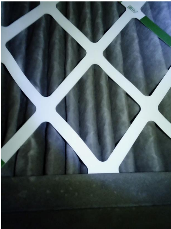
AHU_02 Mixed Main Filter Cleanliness
