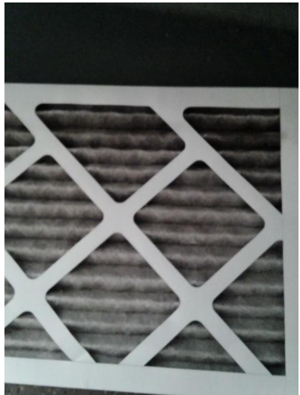
UNIT VENTILATOR Outdoor Main Filter Cleanliness
