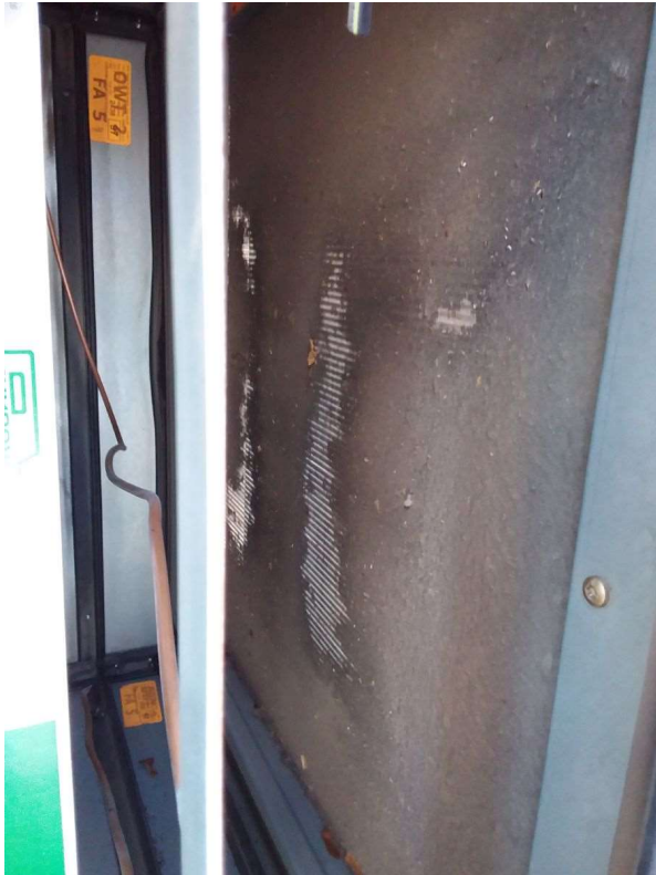
RTU_A1 Heating Coils
