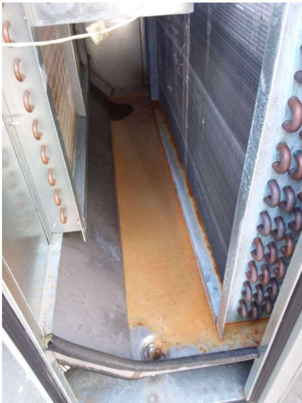
DOAS_C1 Drain Pans
