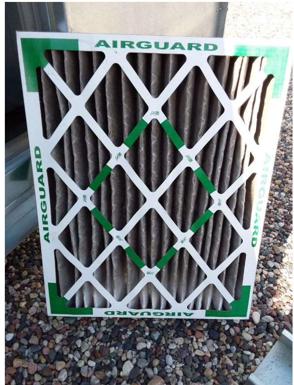
MAU-1 Outdoor Main Filter Cleanliness
