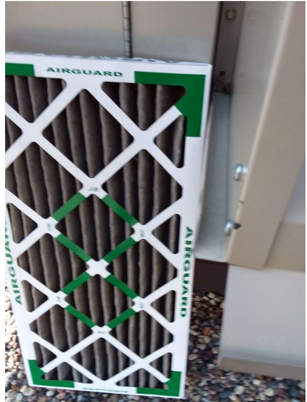
RTU_A1 Mixed Main Filter Cleanliness
