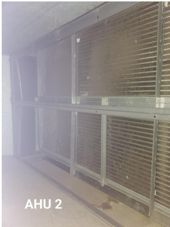
AHU 02 Heating Coils
