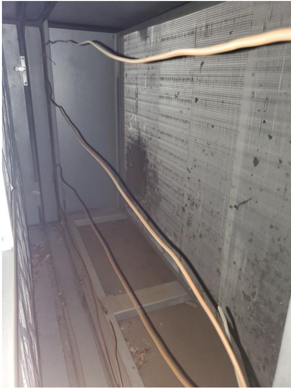
AHU-07 Heating Coils
