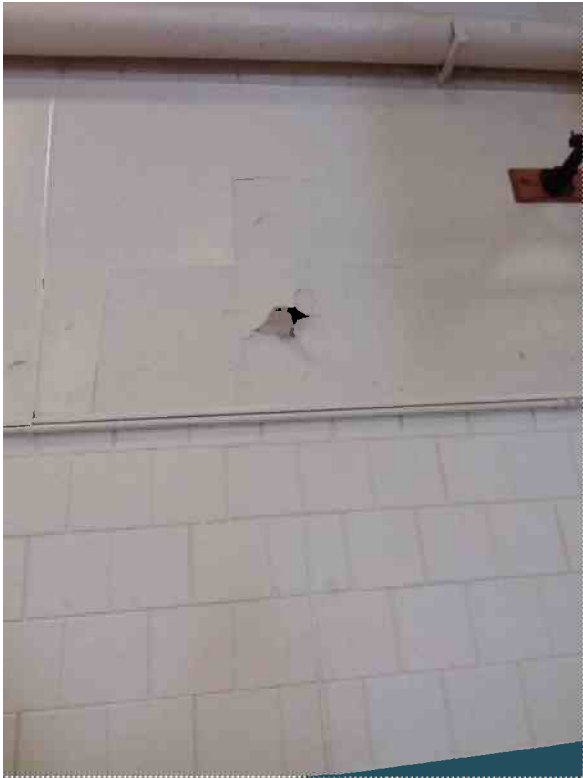
2104 GYMNASIUM Bubbling/Peeling Paint
