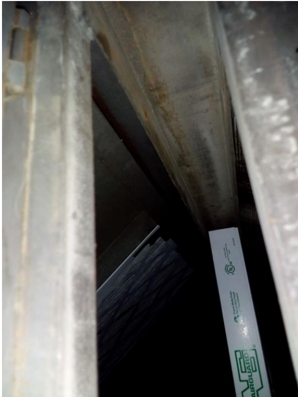
AHU_11 Heating Coils
