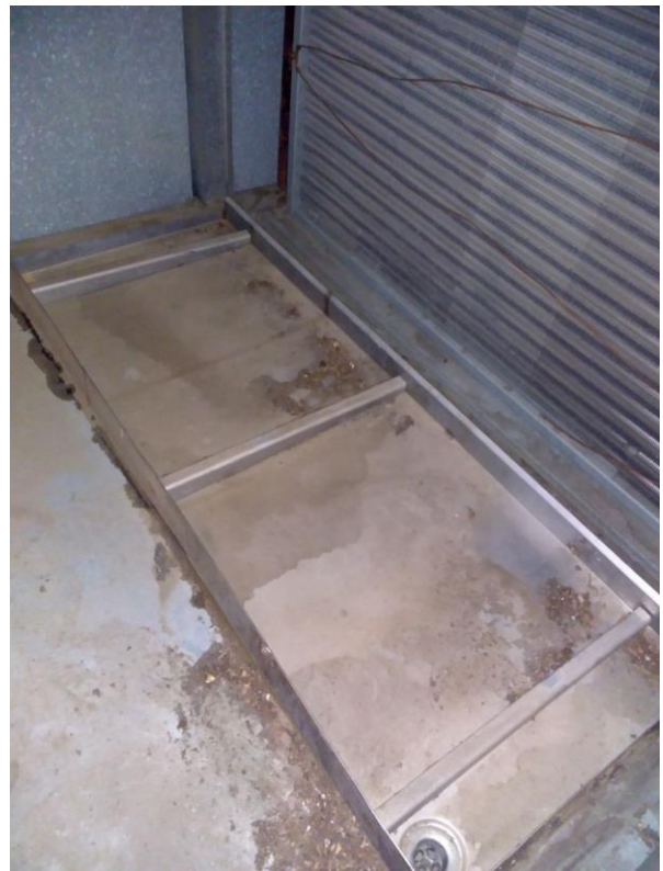
AHU_23 Drain Pans
