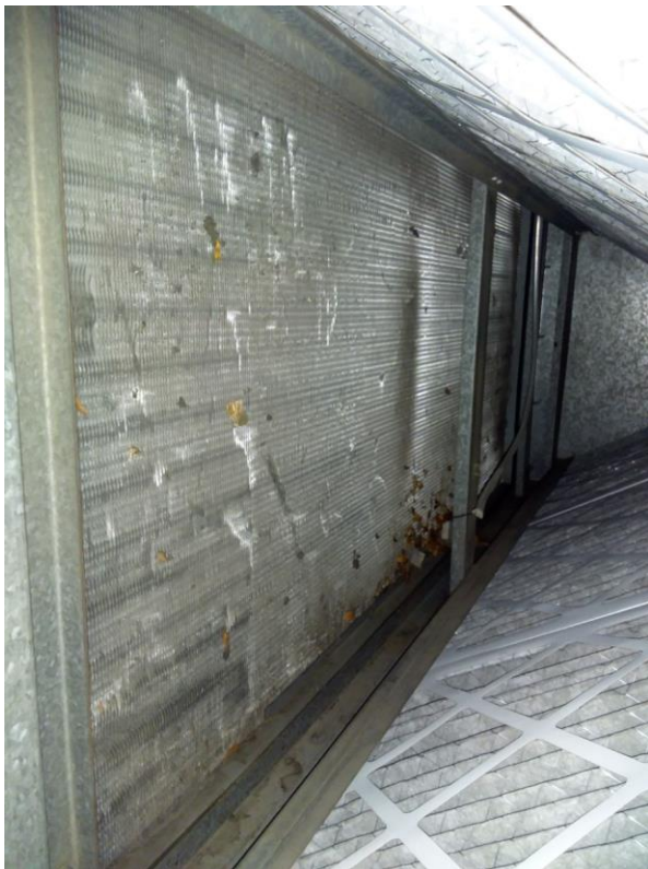
AHU_23 Heating Coils
