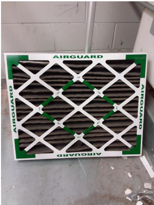
AHU_16 Mixed Main Filter Cleanliness
