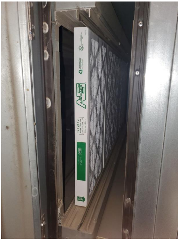
AHU 05 Mixed Main Filter Fit
