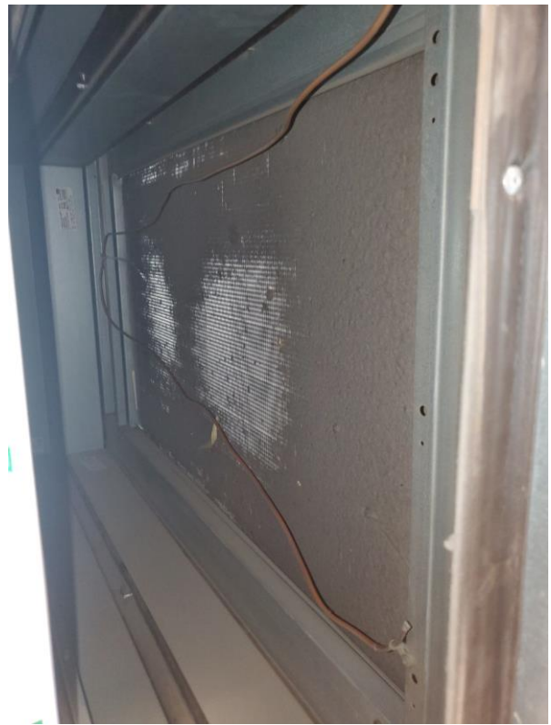
AHU 05 Heating Coils
