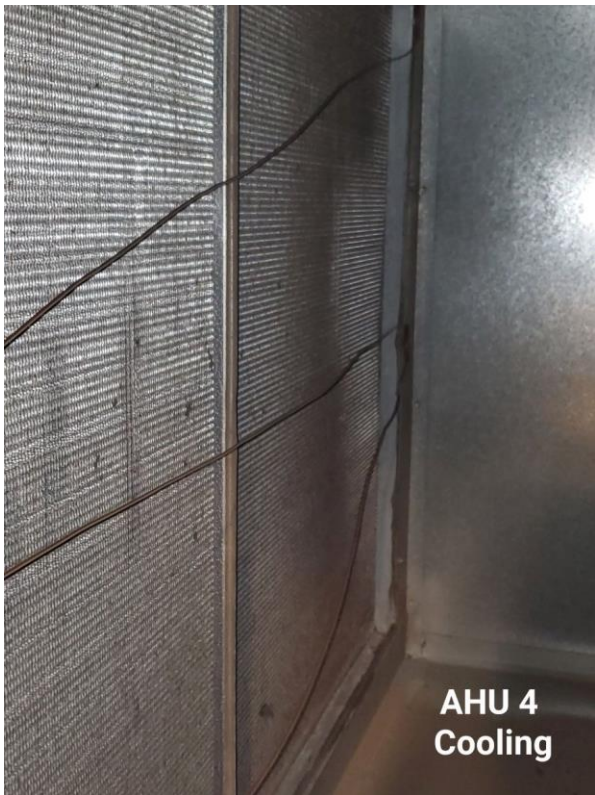
AHU-4 Cooling Coils
