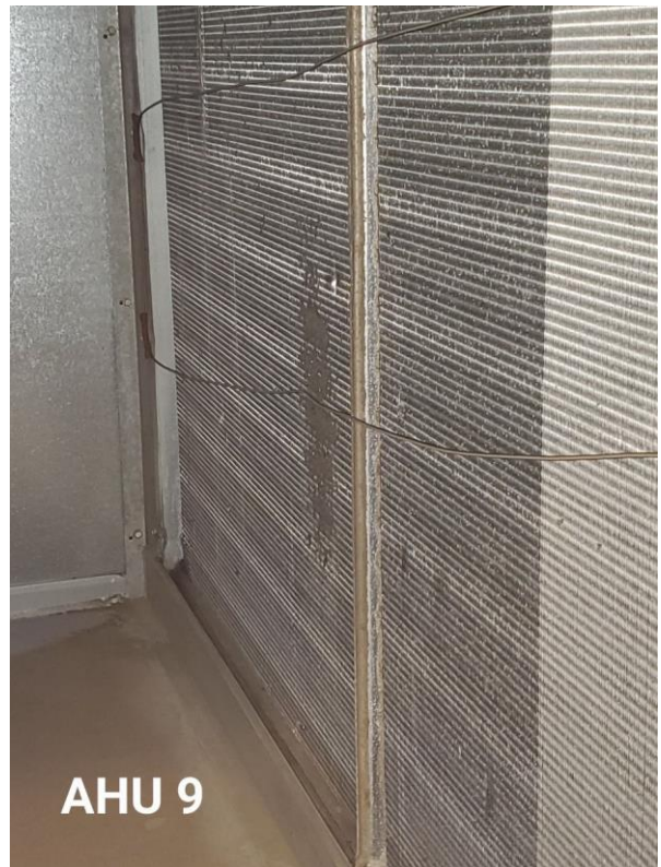
AHU-9 Heating Coils
