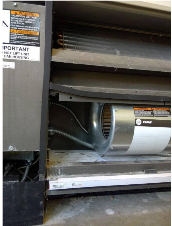
UV-1405 Return Main Filter Installation
