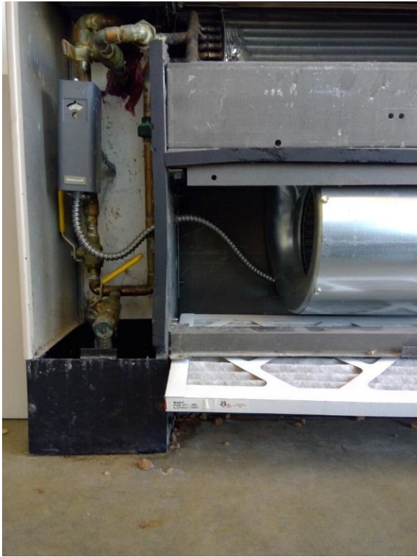
UV-1409 Return Main Filter Installation
