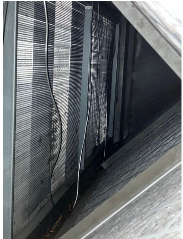
AHU-03 Heating Coils
