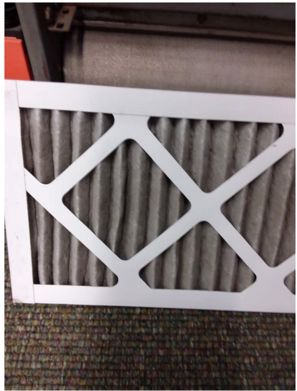
2208 UV Mixed Main Filter Cleanliness
