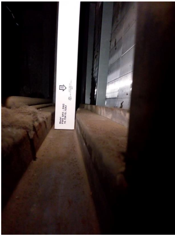
MAU-01 Heating Coils
