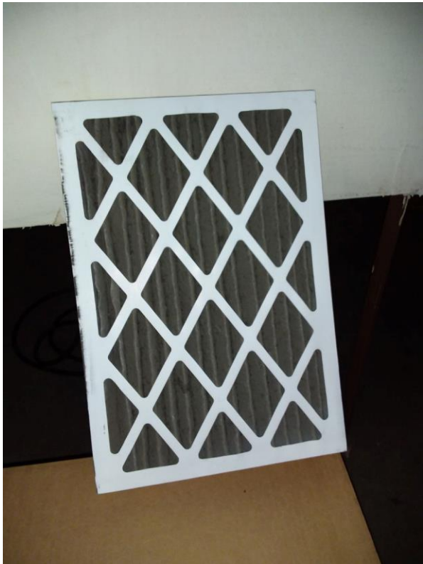
AHU_08 Mixed Main Filter Cleanliness
