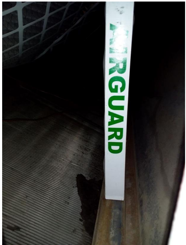
AHU_07 Heating Coils
