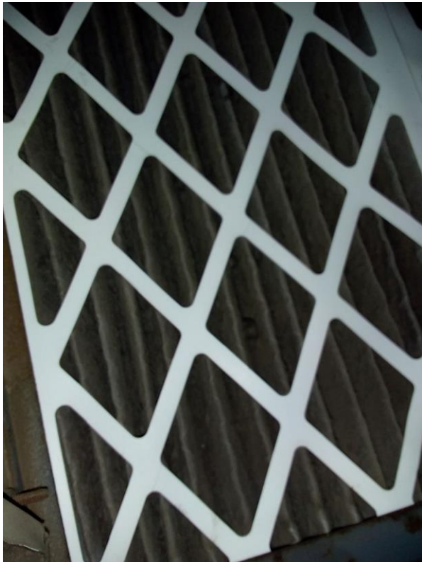
AHU_10 Mixed Main Filter Cleanliness
