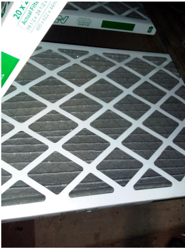
AHU_11 Mixed Main Filter Cleanliness
