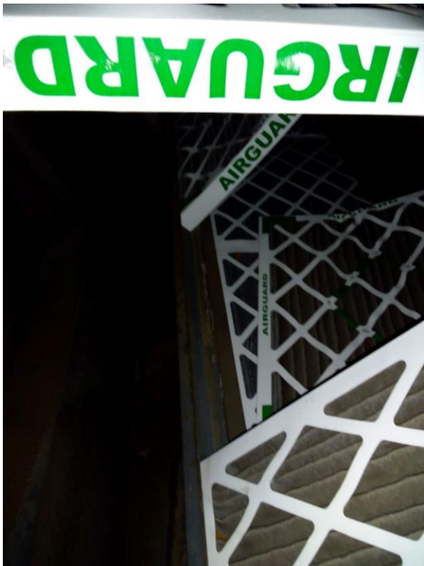
AHU_09 Mixed Main Filter Fit
