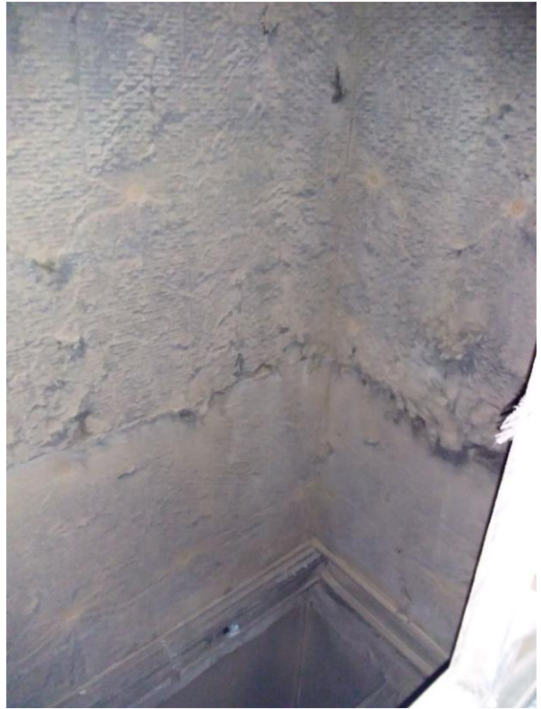
AHU_07 Interior Ducting
