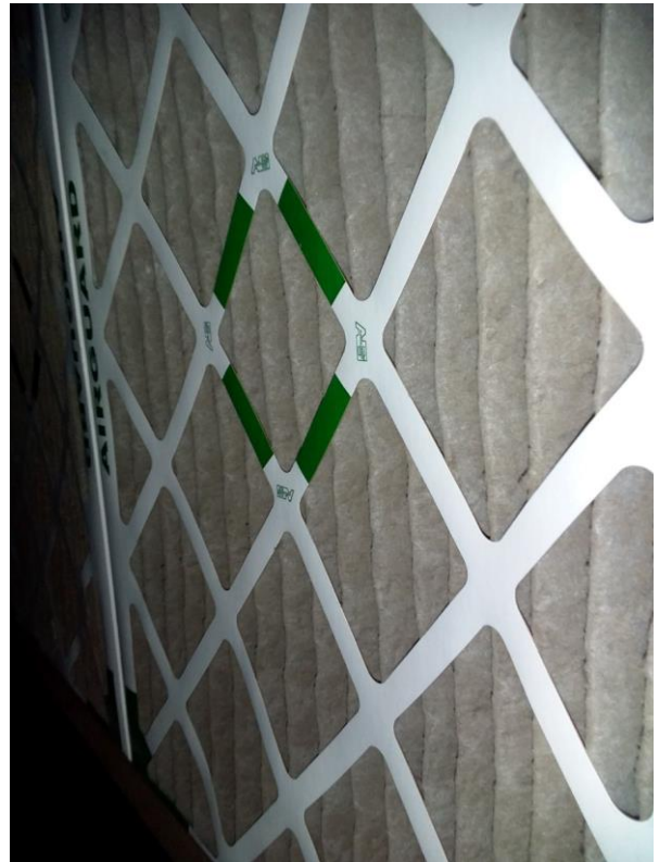
AHU_03 Mixed Main Filter Cleanliness
