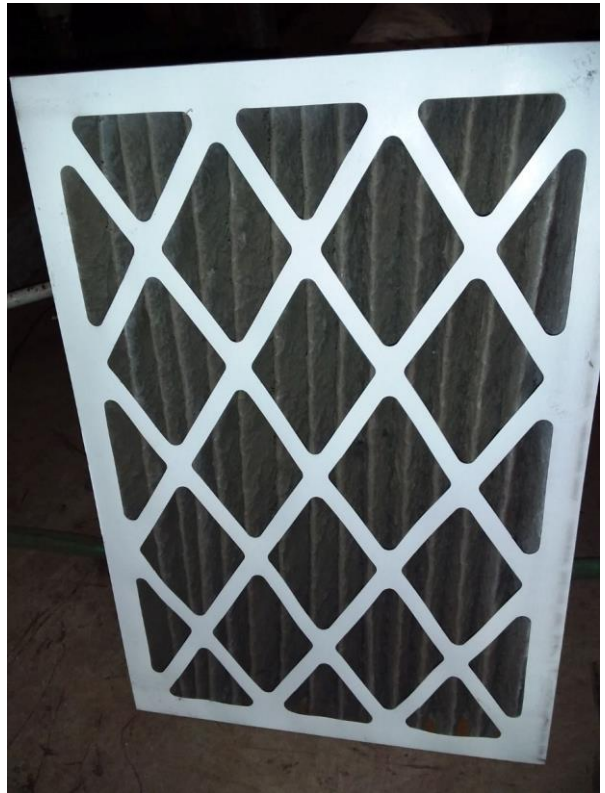
AHU_09 Mixed Main Filter Cleanliness
