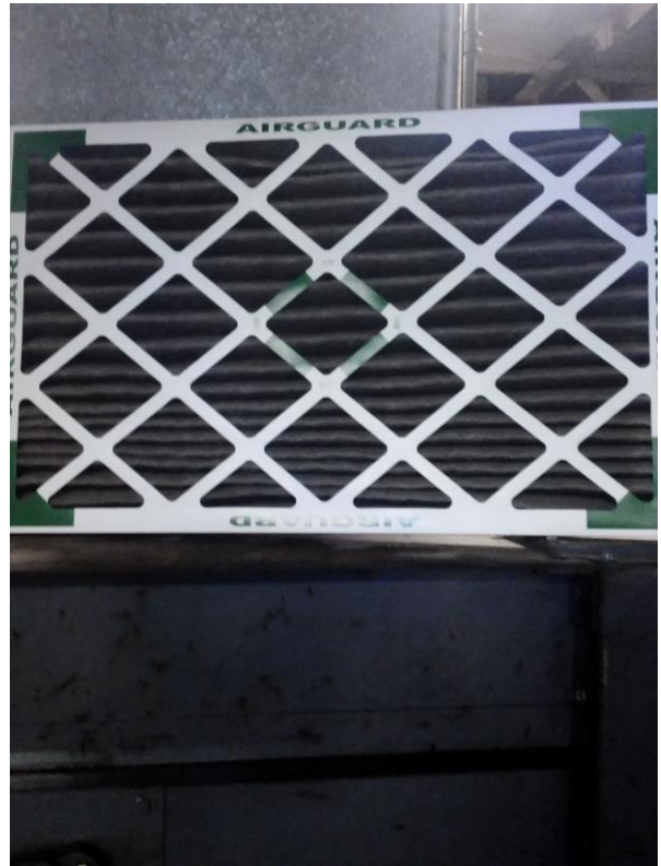
AHU_13 Mixed Main Filter Cleanliness
