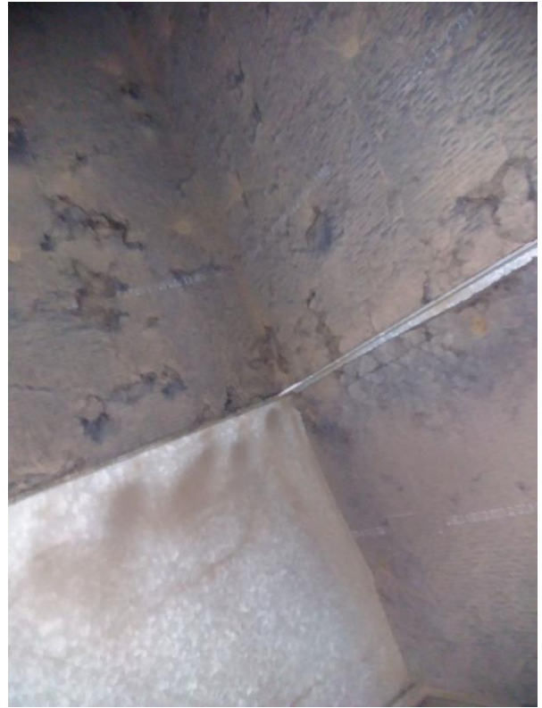
AHU_04 Interior Ducting
