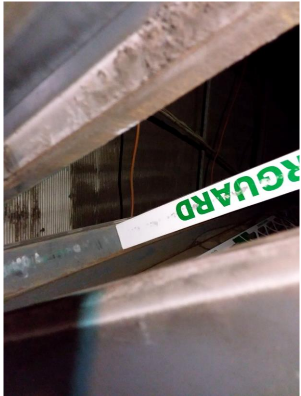
AHU_10 Heating Coils
