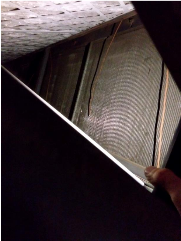
AHU_04 Heating Coils
