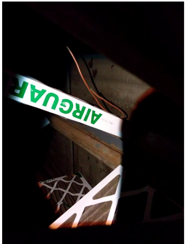
AHU_09 Heating Coils
