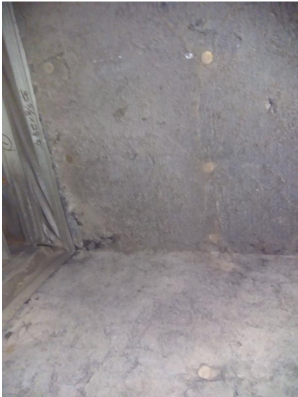
AHU_12 (100% RA) Interior Ducting
