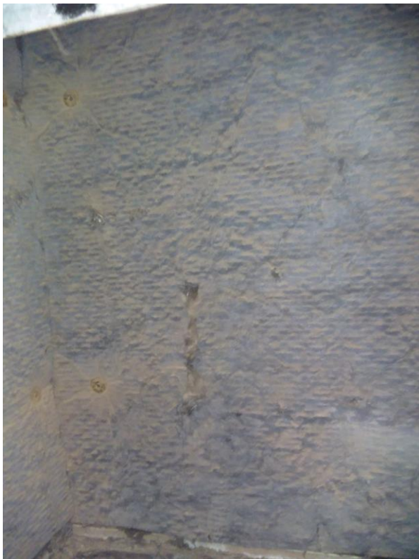
AHU_06 Interior Ducting
