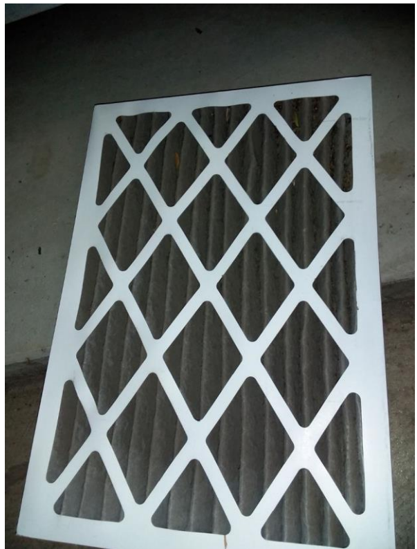
AHU_07 Mixed Pre-Filter Cleanliness
