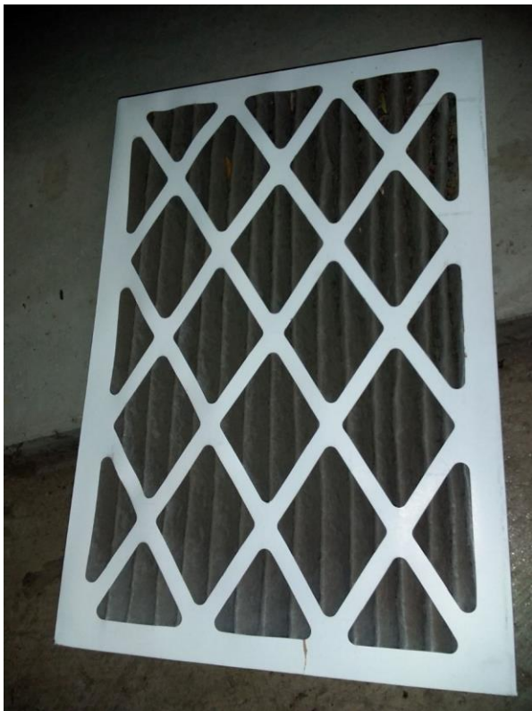
AHU_07 Mixed Main Filter Cleanliness
