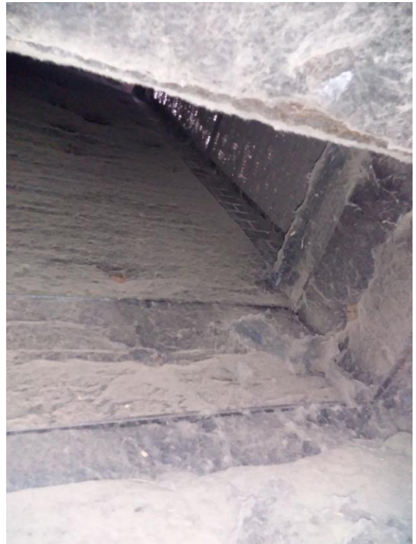
AHU-04 Outdoor Intake
