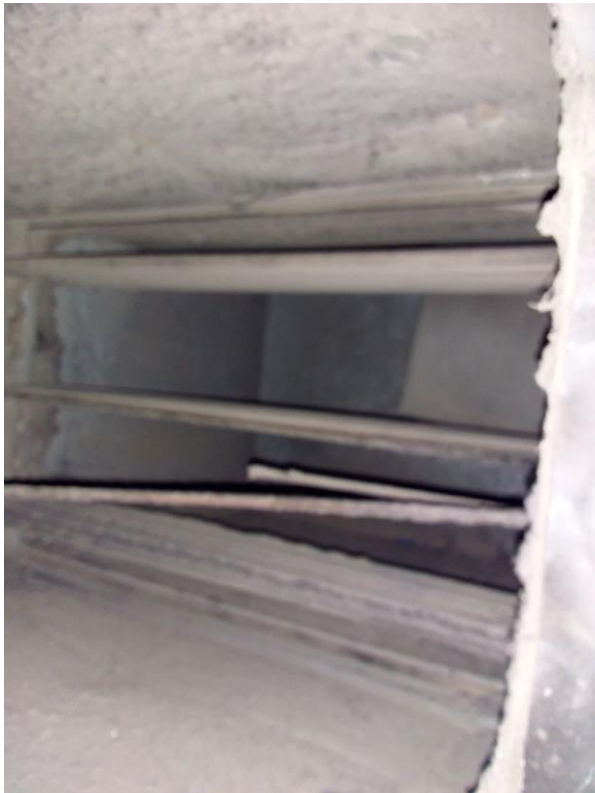
AHU-04 Outside Damper
