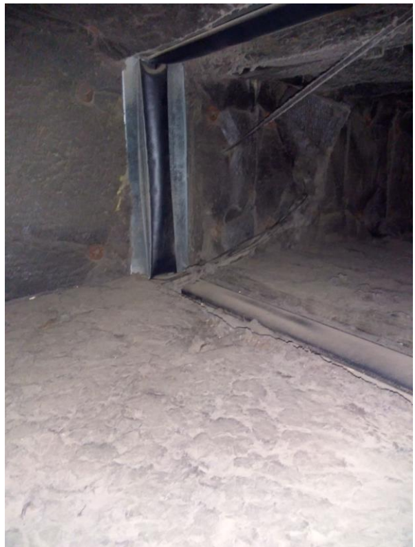
AHU-04 Interior Ducting
