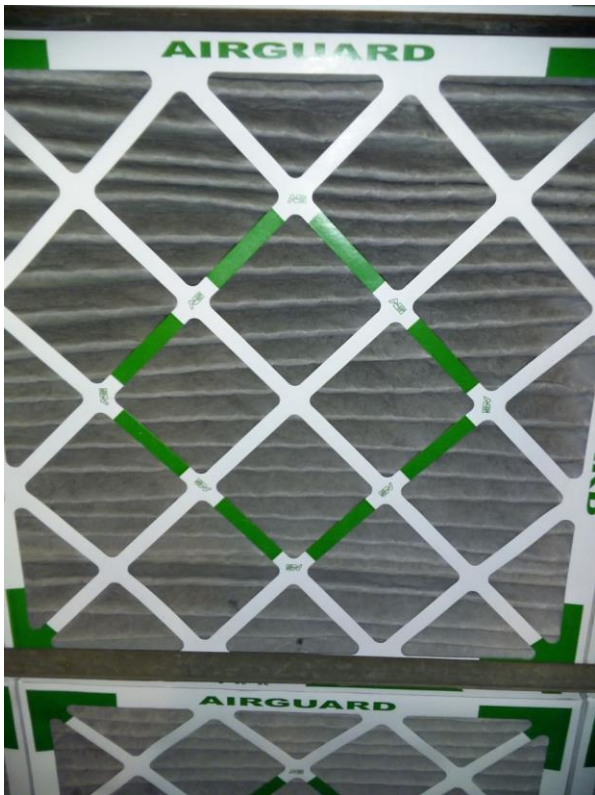
AHU-05 Mixed Main Filter Cleanliness
