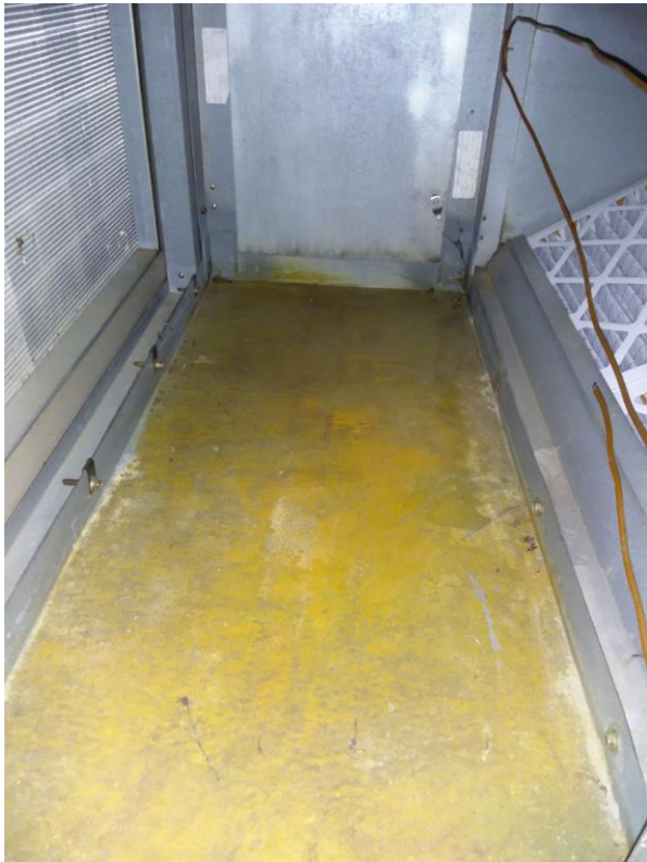
AHU-11 Drain Pans
