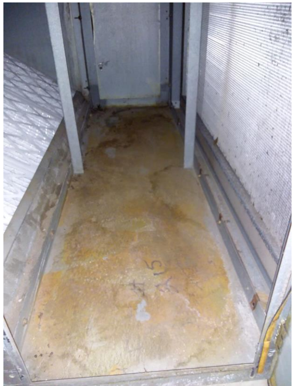
AHU-10 (100% OA) Drain Pans
