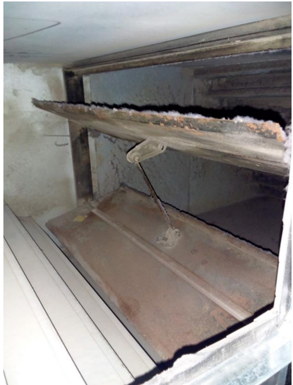
AHU-7 Outside Damper
