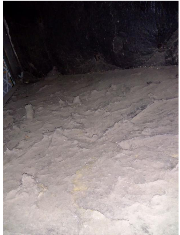
AHU-03 Interior Ducting
