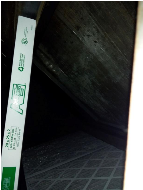
AHU-09 Heating Coils
