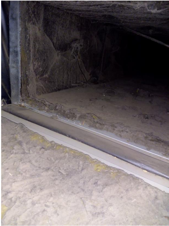
AHU-03 Interior Ducting
