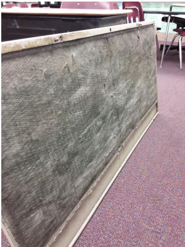
1208 UV Interior Ducting
