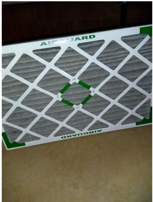
AHU-06 Mixed Main Filter Cleanliness
