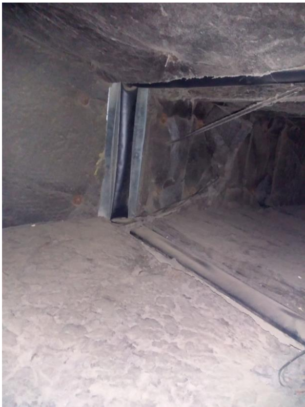
AHU-04 Interior Ducting
