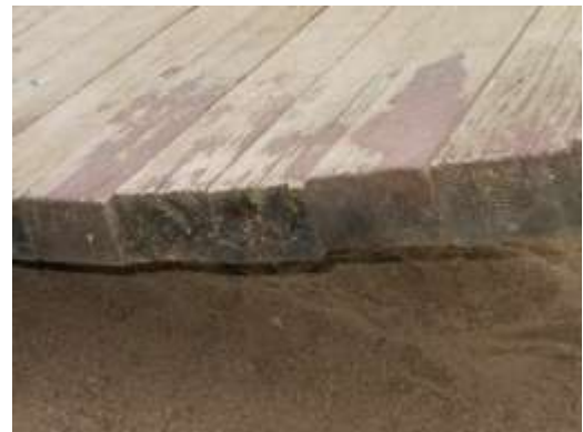
Deteriorating wood at clatter bridge.
