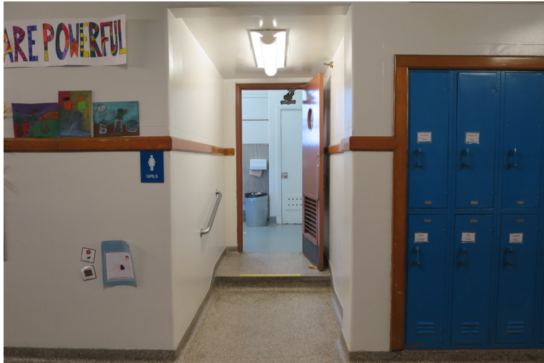
Inaccessible restrooms (all floors)
