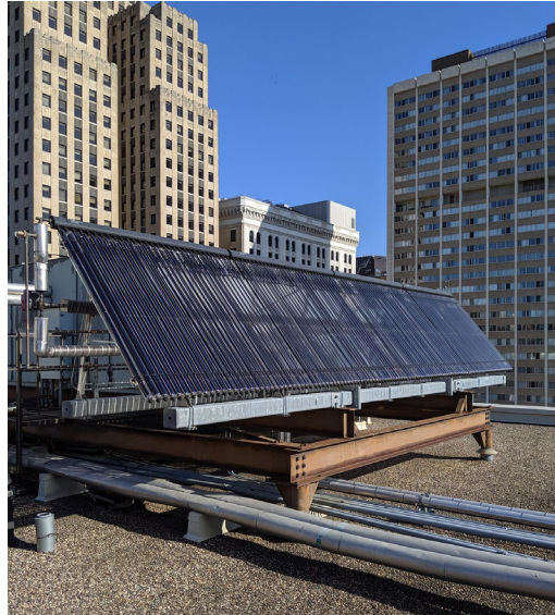
Creative Arts Secondary School Thermal Solar Array
