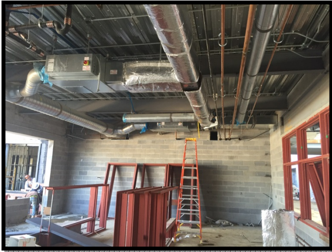
Overhead Electrical, Mechanical and Plumbing
