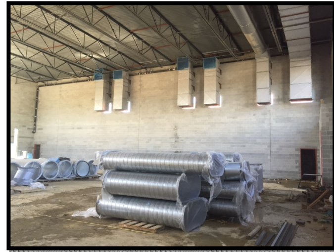
HVAC Duct at Gym
