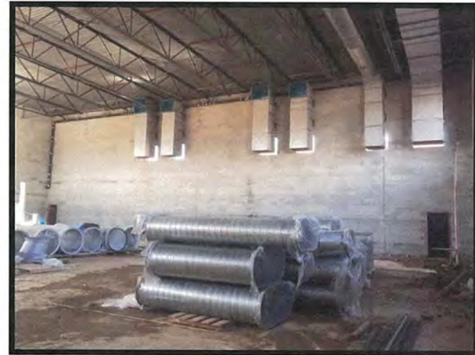
HVAC Duct at Gym
