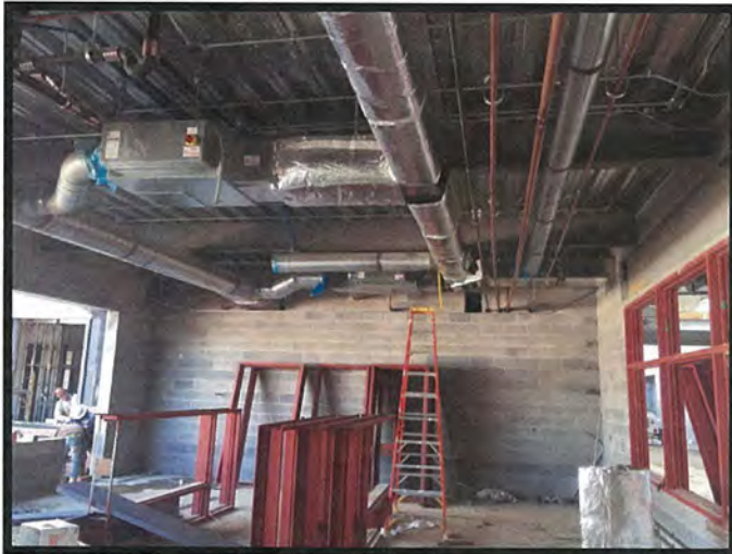
Overhead Electrical, Mechanical and Plumbing
