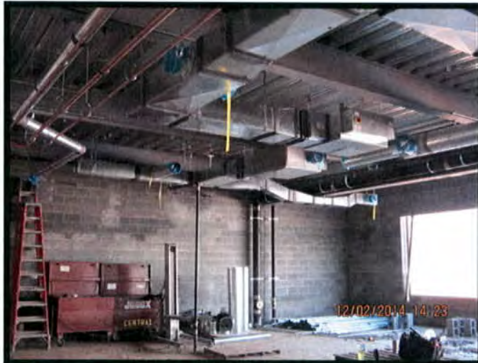
HVAC Duct and Plumbing
