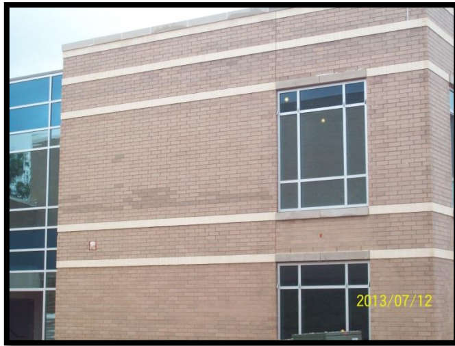
Brick Staining - BEFORE
