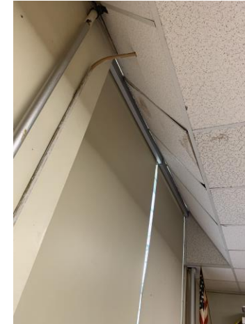
Typical Ceiling Condition
