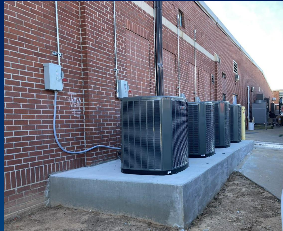
New HVAC Equipment
