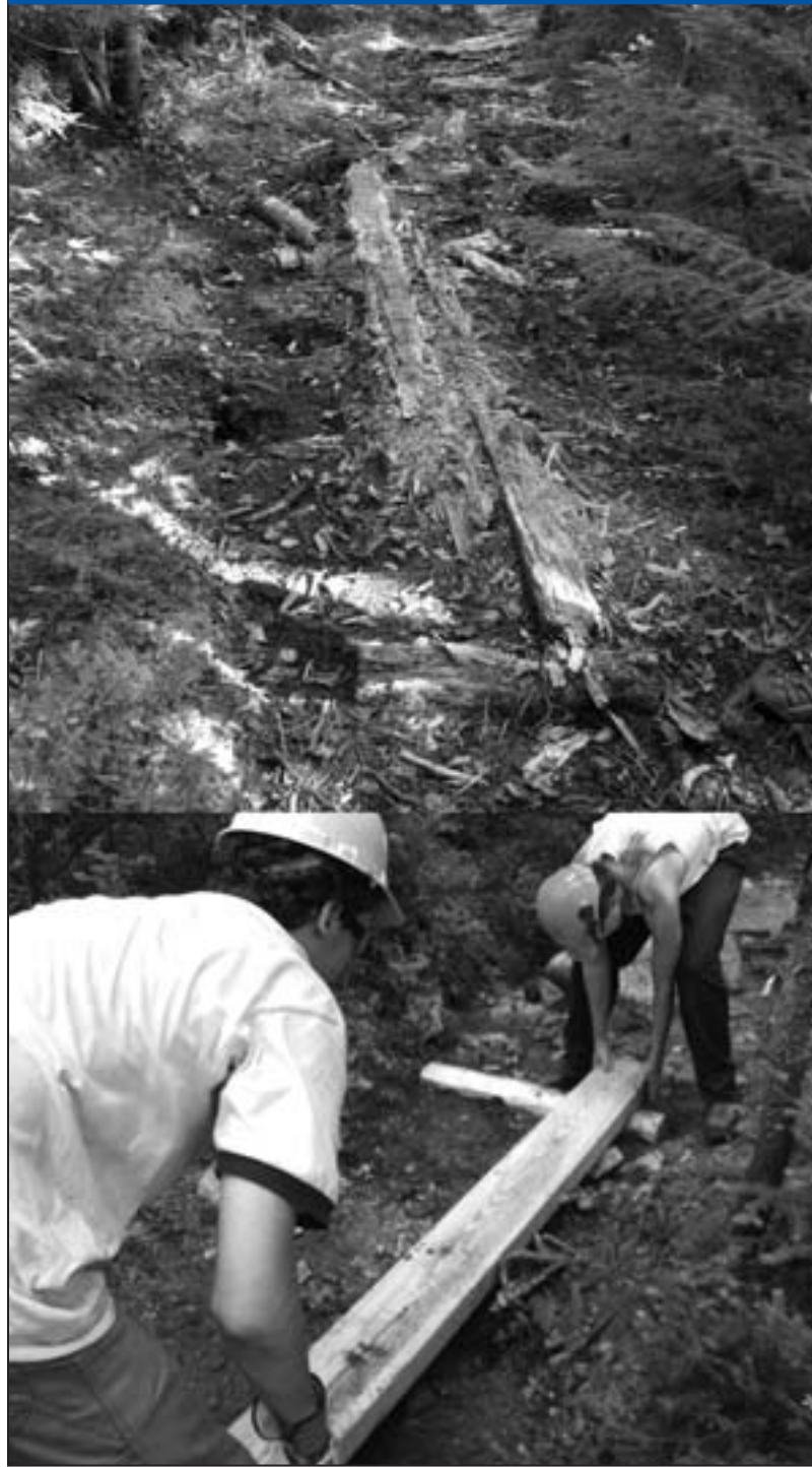
Top: One of the many bog bridges in disrepair along the Nancy Pond Trail in 2009 (photo courtesy of Steve Dittmann). Bottom: Taylor Barker and Tyler Brown installing a new bridge in 2010.
