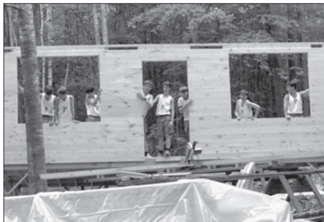
"Veteran counsellor Dave Ryder, with a corps of campers, counsellors, and some alumni, worked his magic and continued to meet Pasquaney's building needs. Over the summers of 1992 and 1993 they constructed a council work office, The Owen S. Lindsay Centennial Hall, between the library and the Alumni House."
