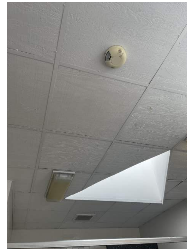
Image 2.3.4 Restroom ceiling. Taken on 04/27/2022 by Belli Architectural Group.
