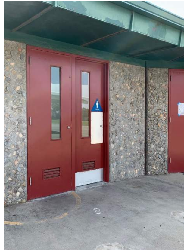
Image 2.2.3 Non-accessible doors and threshold issues. Taken on 04/27/2022 by Belli Architectural Group.
