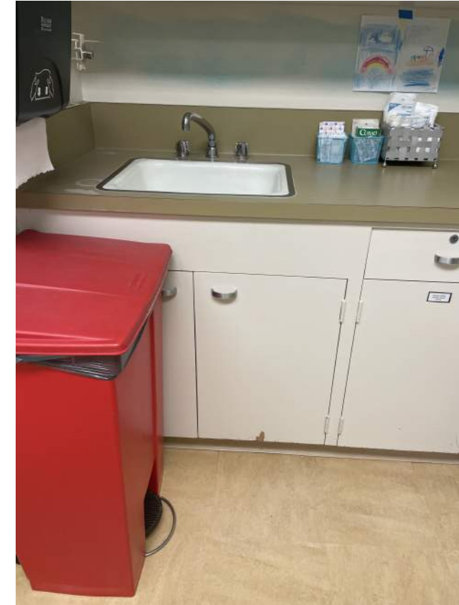
Image 2.4.3 Non-compliant sinks. Taken on 04/27/2022 by Belli Architectural Group.
