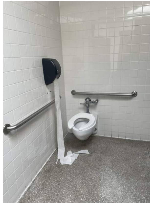
Image 2.4.2 Non-compliant accessories. Taken on 04/27/2022 by Belli Architectural Group.
