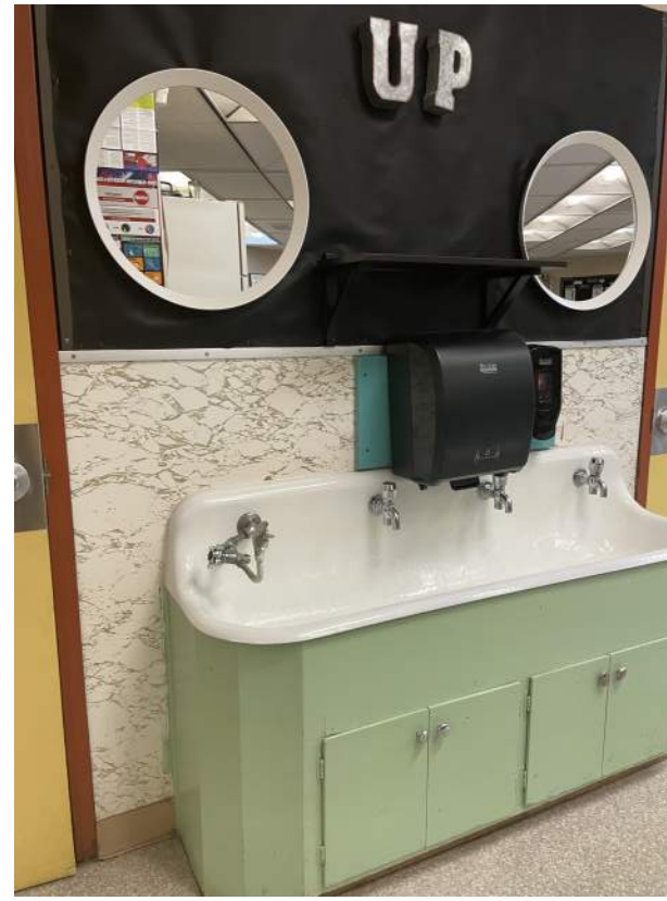
Image 2.3.8 Kindergarten sized plumbing fixtures used by staff. Taken on 04/27/2022 by Belli Architectural Group.
