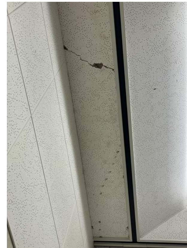
Image 2.3.3 Damaged ceiling panels. Taken on 04/27/2022 by Belli Architectural Group.
