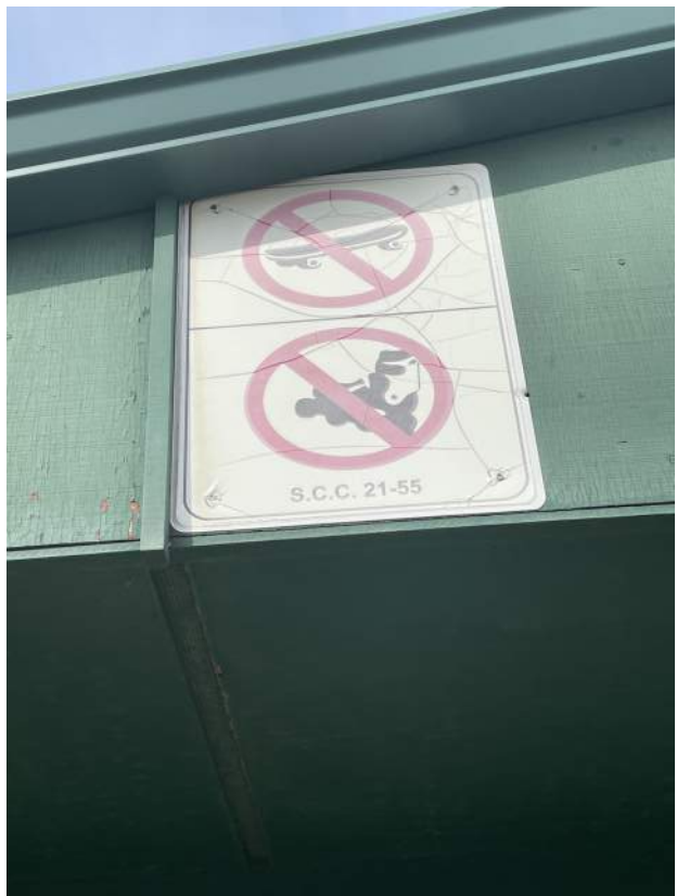
Image 2.2.2 Broken signage. Taken on 04/27/2022 by Belli Architectural Group.
