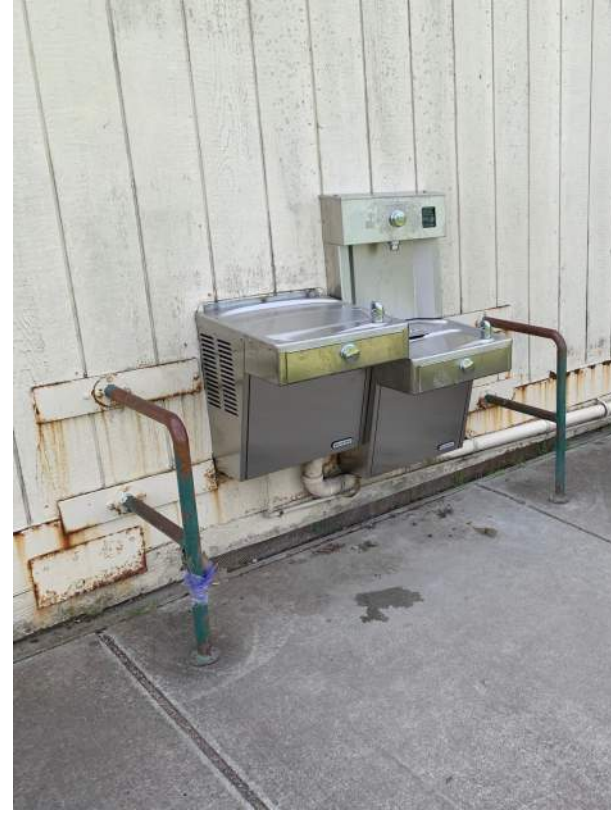
Image 2.2.3 Rust present at relocatable classrooms. Taken on 04/27/2022 by Belli Architectural Group.
