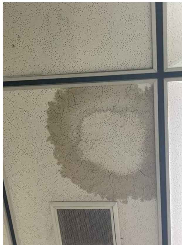
Image 2.3.2 Evidence of leaks in ceiling panels. Taken on 04/27/2022 by Belli Architectural Group.
