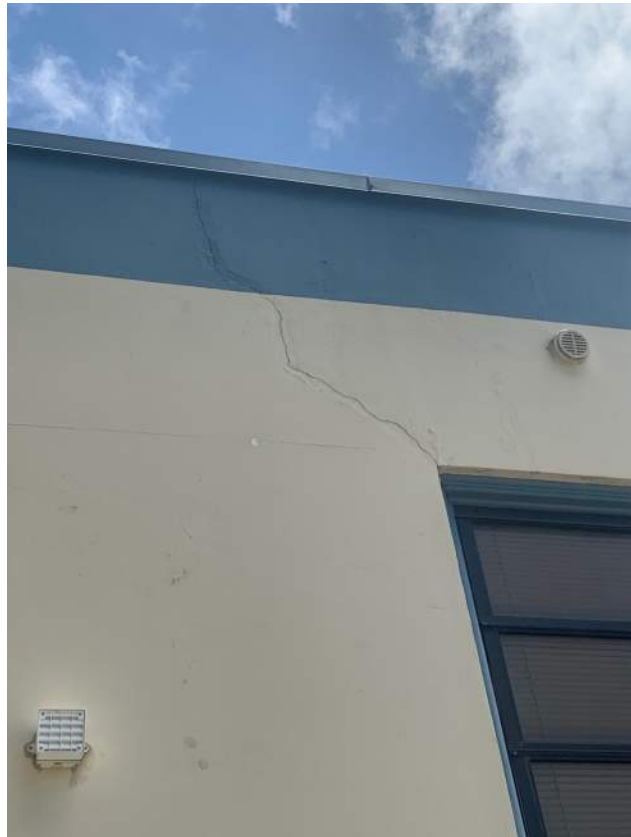
Image 2.2.4 Building A, exterior cracks. Taken on 05/02/2022 by Belli Architectural Group.
