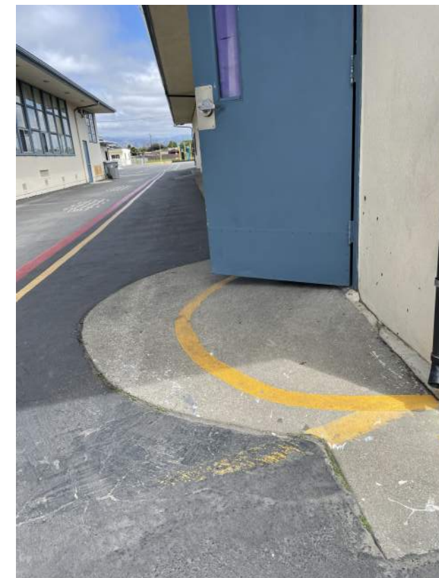
Image 2.2.14 Non-accessible entry at Building F. Taken on 05/02/2022 by Belli Architectural Group.
