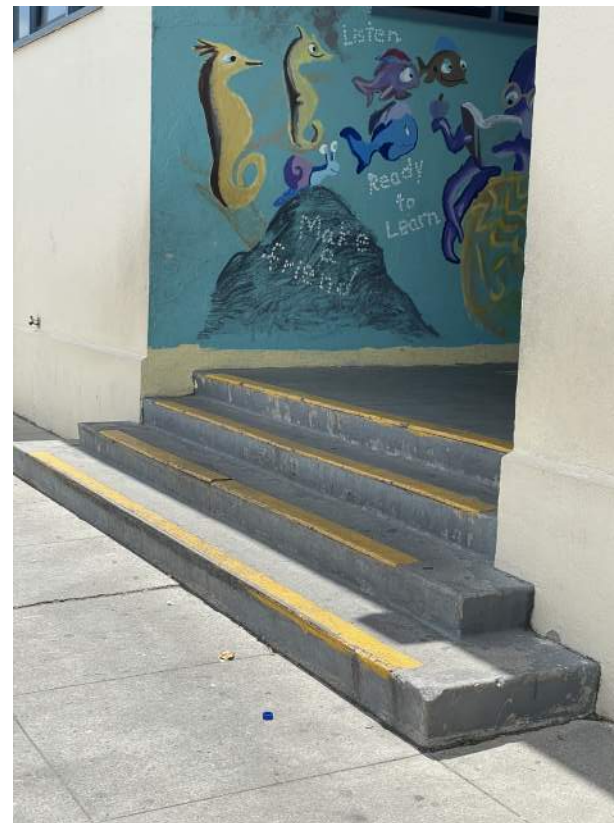
Image 2.1.4 Non-accessible stairs. Taken on 04/26/2022 by Belli Architectural Group.
