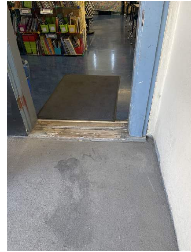
Image 2.2.8 Non-compliant door threshold at building B. Taken on 05/02/2022 by Belli Architectural Group.
