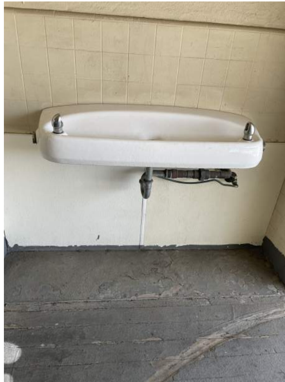
Image 2.1.7 Non-accessible drinking fountain. Taken on 05/02/2022 by Belli Architectural Group.
