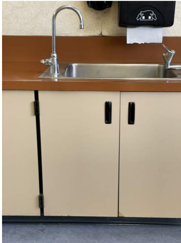
Image 2.4.3 Non-ADA compliant classroom sink. Taken on 05/02/2022 by Belli Architectural Group.
