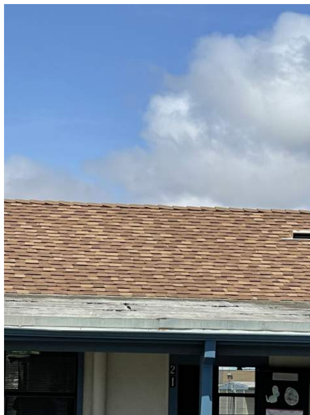
Image 2.2.5 Building B, old, damaged roof at outdoor covered walkway. Taken on 05/02/2022 by Belli Architectural Group.
