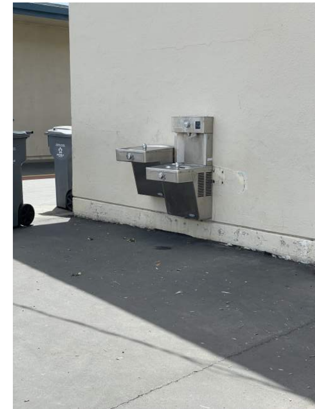
Image 2.4.2 Drinking fountain missing cane detection rails. Taken on 05/02/2022 by Belli Architectural Group.
