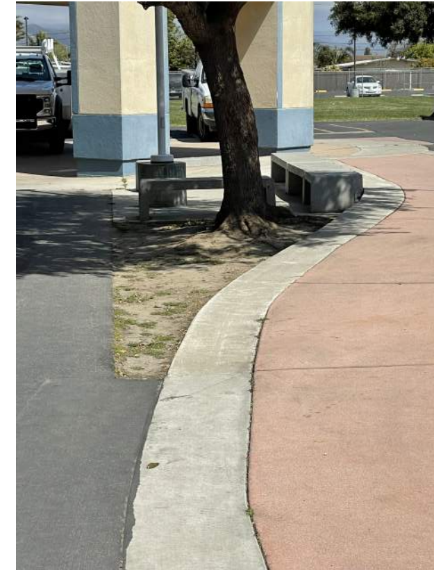
Image 2.1.5 Trip hazards present with uneven walking surfaces. Taken on 05/02/2022 by Belli Architectural Group.
