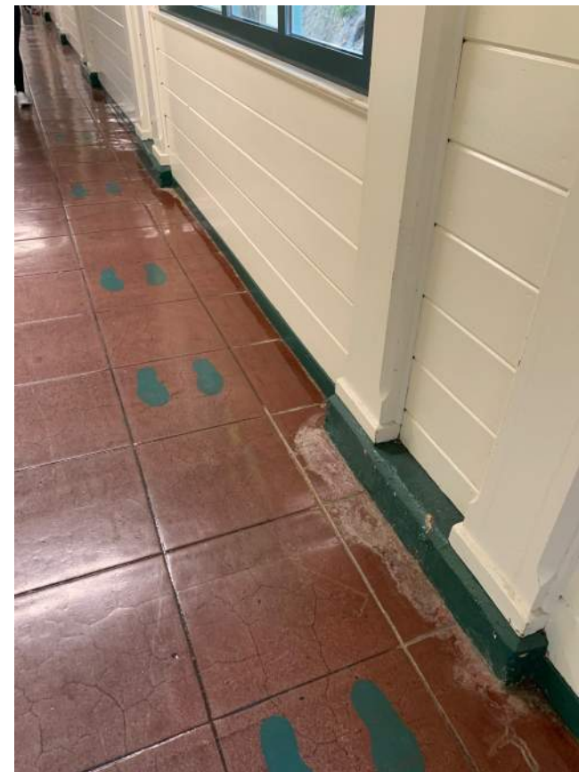
Image 2.2.1 Water intrusion in hallway. Taken on 04/27/2022 by Belli Architectural Group.
