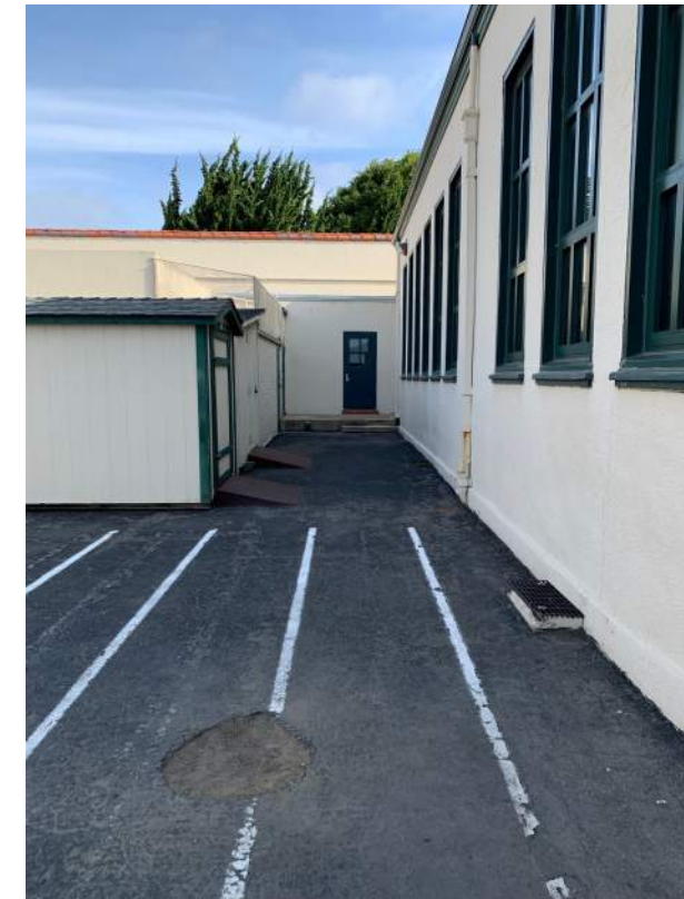
Image 2.1.4 Uneven asphalt surfaces. Taken on 04/27/2022 by Belli Architectural Group.
