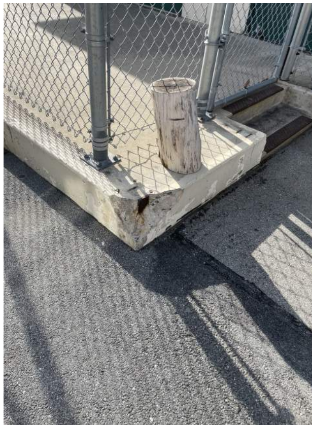
Image 2.1.6 Spalling at curb. Taken on 04/27/2022 by Belli Architectural Group.
