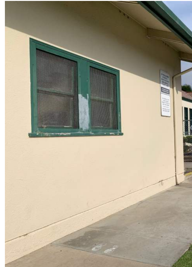
Image 2.2.5 Damaged windows. Taken on 04/27/2022 by Belli Architectural Group.
