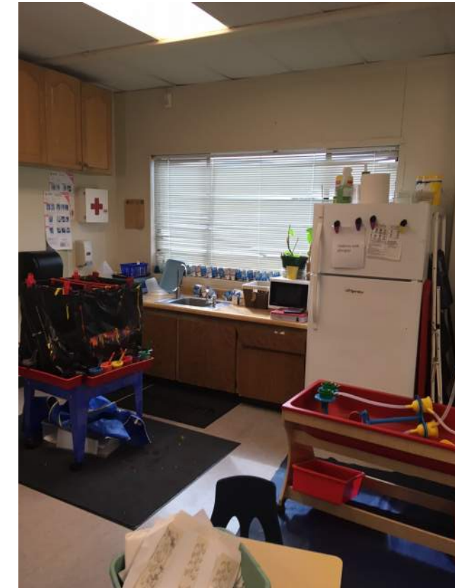
Image 2.3.10 Preschool. Non-compliant sink. Taken on 04/27/2022 by Belli Architectural Group.
