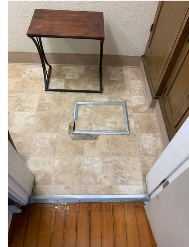
Image 2.3.9 Patched sheet vinyl flooring. Taken on 04/27/2022 by Belli Architectural Group.
