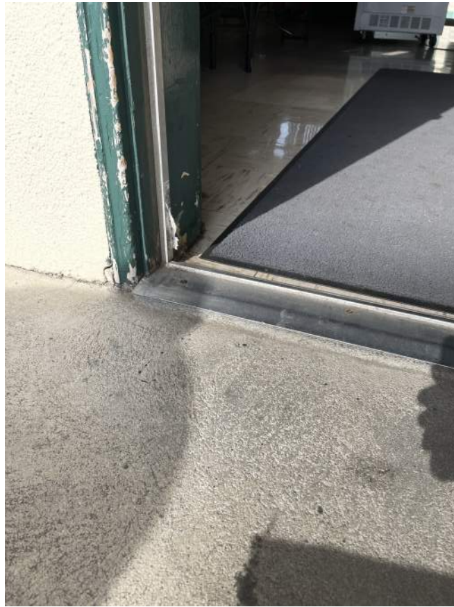
Image 2.2.4 Damaged door frames. Taken on 04/27/2022 by Belli Architectural Group.
