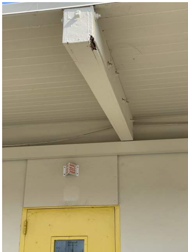
Image 2.2.2 Dry rot at eave condition. Taken on 05/02/2022 by Belli Architectural Group.
