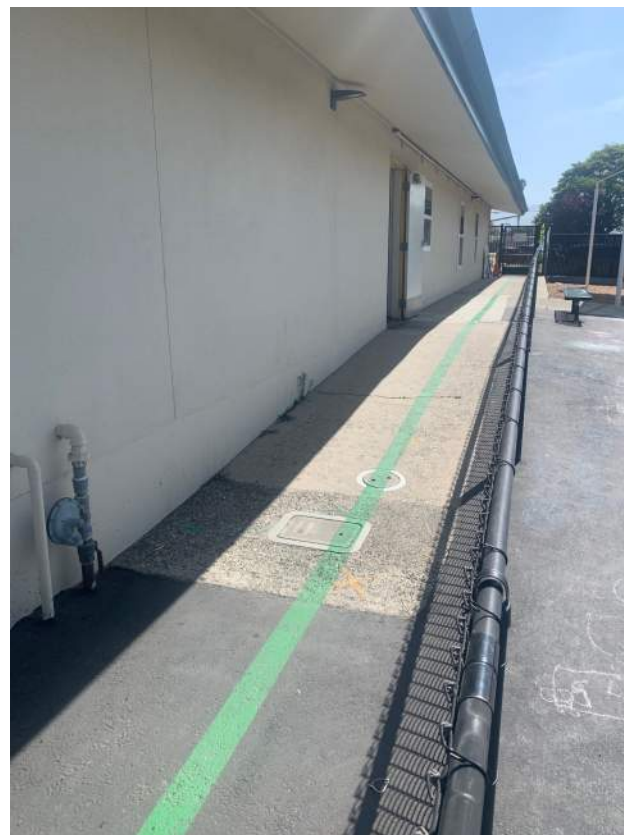
Image 2.1.1 Damaged walkways. Taken on 05/02/2022 by Belli Architectural Group.
