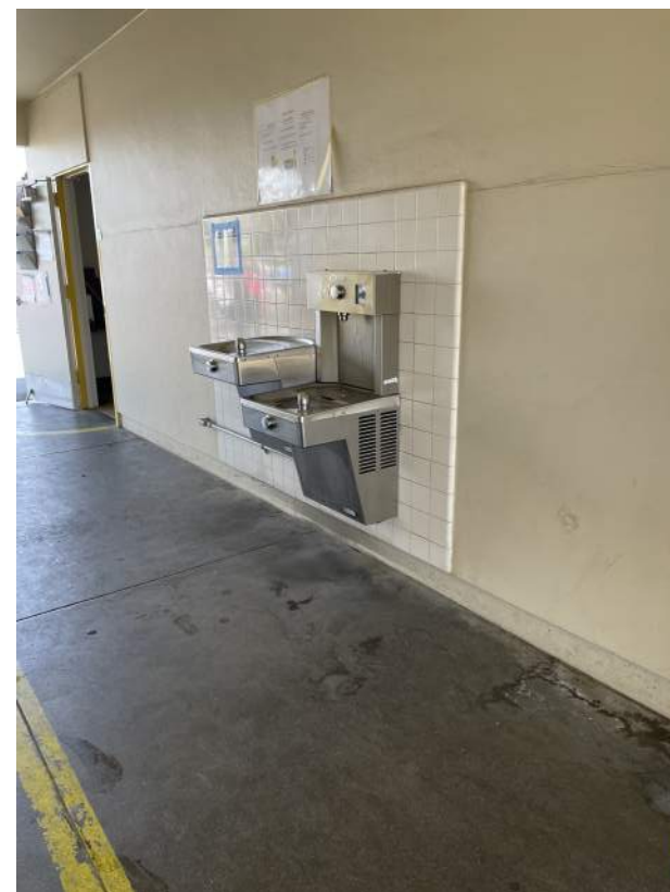
Image 2.4.3 Drinking fountain missing cane detection rails. Taken on 05/02/2022 by Belli Architectural Group.
