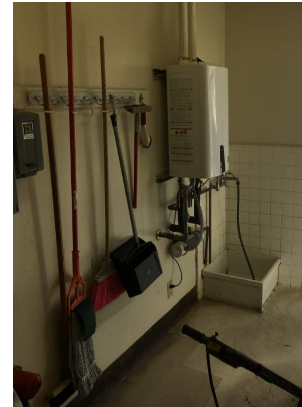
Image 2.3.8 Janitorial room. Taken on 05/02/2022 by Belli Architectural Group.
