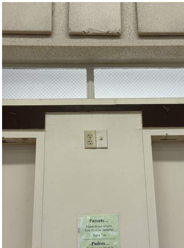
Image 2.3.4 Broken acoustic panel at MPR. Taken on 04/27/2022 by Belli Architectural Group.
