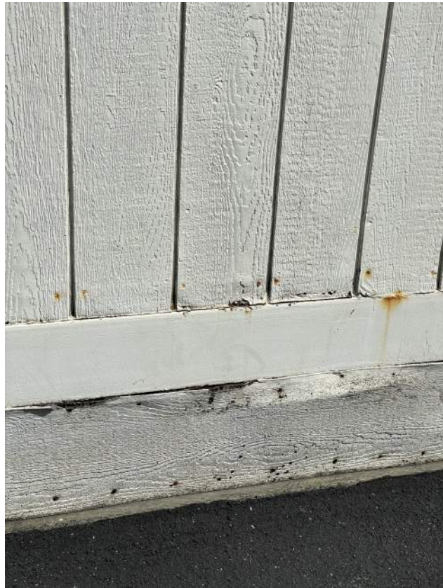
Image 2.2.5 Rust present at relocatable classrooms. Taken on 04/27/2022 by Belli Architectural Group.
