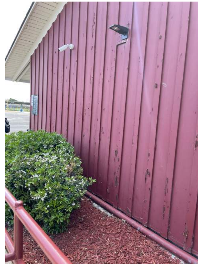
Image 2.2.1 Exterior paint peeling. Taken on 04/27/2022 by Belli Architectural Group.
