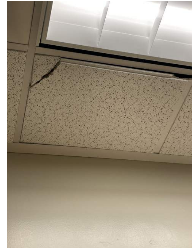
Image 2.3.1 Broken ceiling panels. Taken on 04/27/2022 by Belli Architectural Group.
