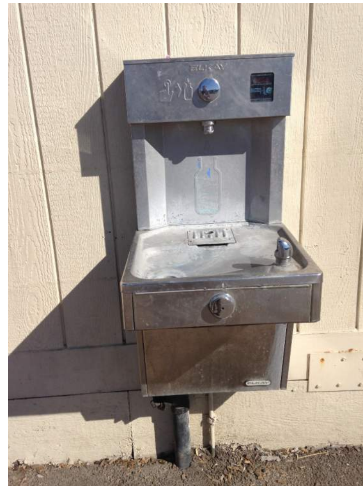
A bottle filler near Classroom 24 in need of replacement.
