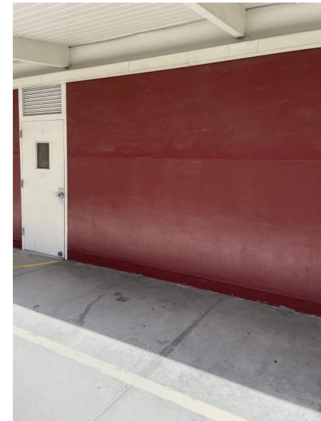
Image 2.2.2 Uneven exterior finishes. Taken on 04/27/2022 by Belli Architectural Group.
