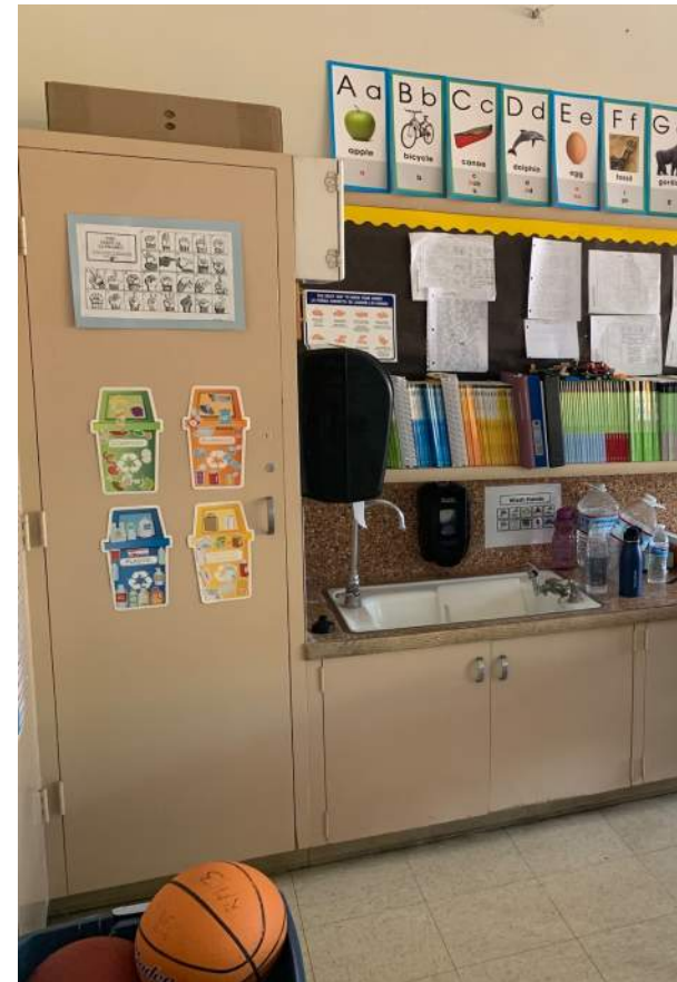
Image 2.4.2 Non-accessible sink. Taken on 04/27/2022 by Belli Architectural Group.
