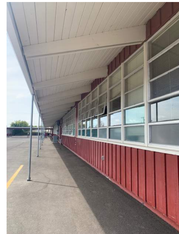
Image 2.2.3 Old, original windows. Taken on 04/27/2022 by Belli Architectural Group.
