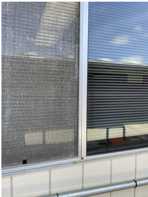
Image 2.2.6 Broken window screen. Taken on 04/27/2022 by Belli Architectural Group.
