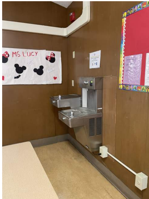
Image 2.4.1 Missing cane detection rails. Taken on 04/27/2022 by Belli Architectural Group.
