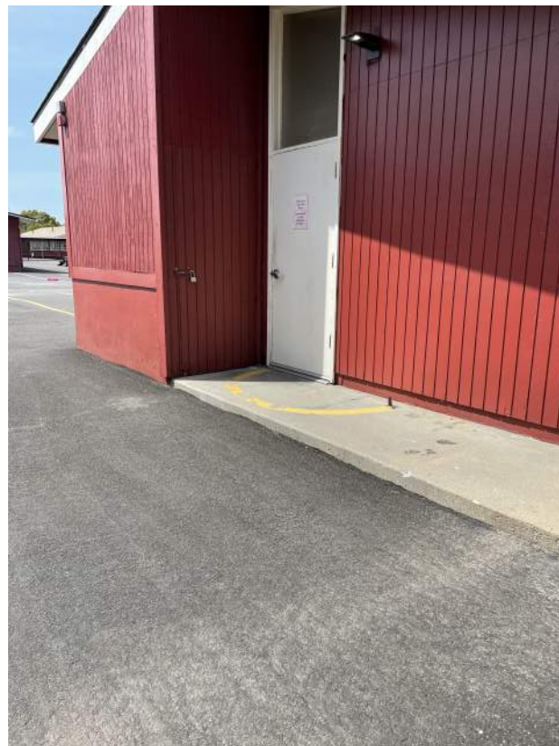
Image 2.1.1 Non-ADA compliant door landing. Taken on 04/27/2022 by Belli Architectural Group.
