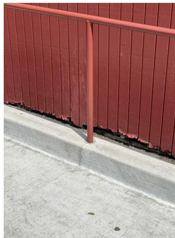
Image 2.2.3 Exterior dry rot. Taken on 04/27/2022 by Belli Architectural Group.
