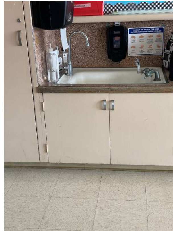
Image 2.3.7 Non-accessible classroom sink. Taken on 04/27/2022 by Belli Architectural Group.
