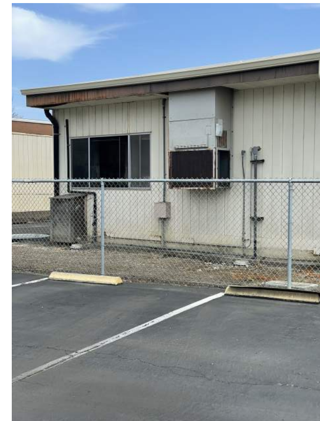
Image 2.2.2 Rust and dry rot at relocatable building. Taken on 04/27/2022 by Belli Architectural Group.
