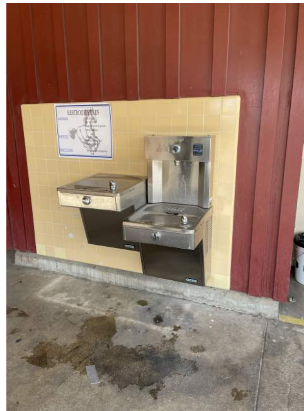
Image 2.4.1 Drinking fountains missing cane detection rails. Taken on 04/27/2022 by Belli Architectural Group.
