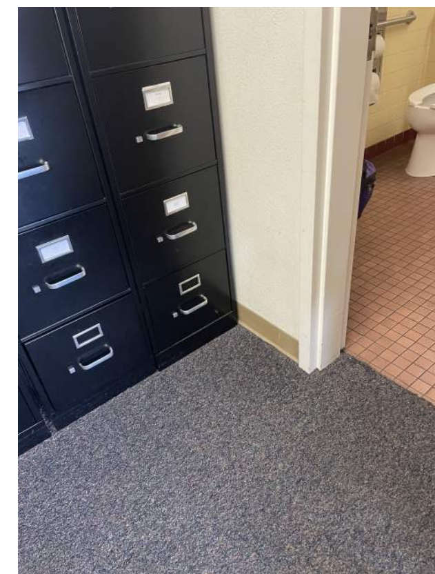
Image 2.3.4 Missing threshold. Taken on 04/27/2022 by Belli Architectural Group.
