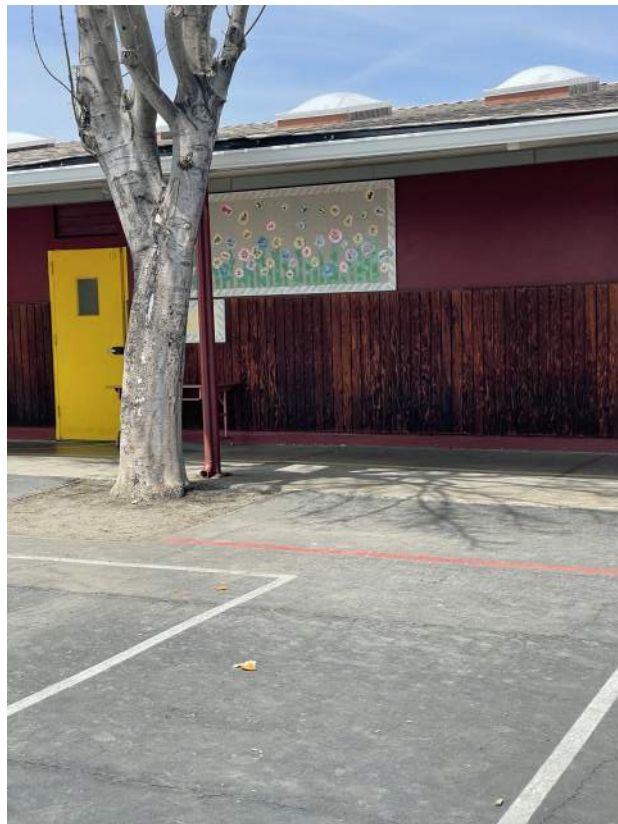
Image 2.2.1 Sagging roof at permanent building. Taken on 04/27/2022 by Belli Architectural Group.
