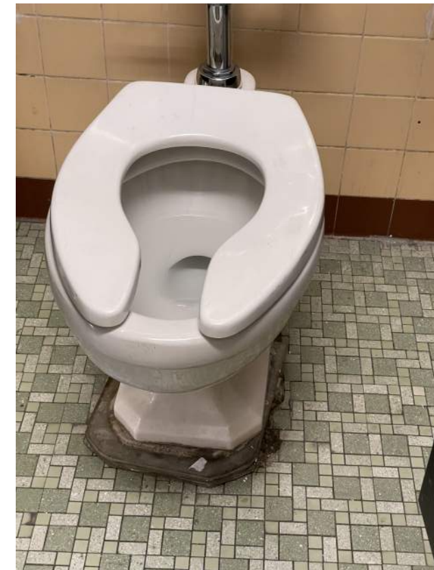
Image 2.3.9 Incorrectly installed water closet. Taken on 04/27/2022 by Belli Architectural Group.
