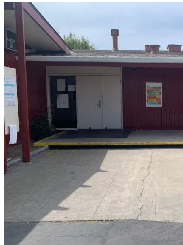
Image 2.1.3 Cracks in walkways. Taken on 04/27/2022 by Belli Architectural Group.
