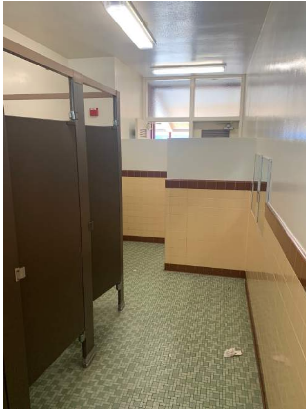
Image 2.4.1 Non-accessible restrooms. Taken on 04/27/2022 by Belli Architectural Group.
