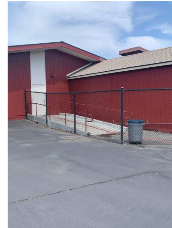
Image 2.1.5 MPR accessible entry at back of building. Taken on 04/27/2022 by Belli Architectural Group.
