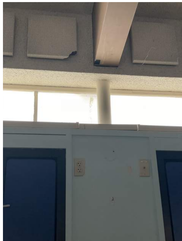
Image 2.3.6 Broken acoustic panel. Taken on 04/27/2022 by Belli Architectural Group.
