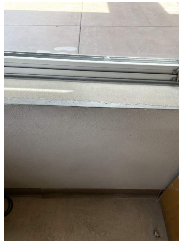
Image 2.3.2 Peeling plaster. Taken on 04/27/2022 by Belli Architectural Group.
