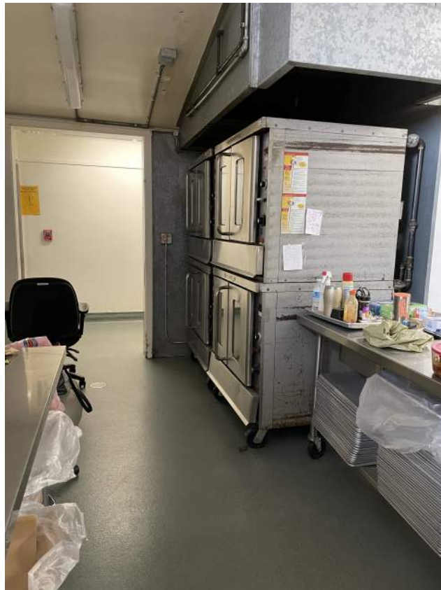
Image 2.3.11 Kinchen equipment. Taken on 06/29/2022 by Belli Architectural Group.
