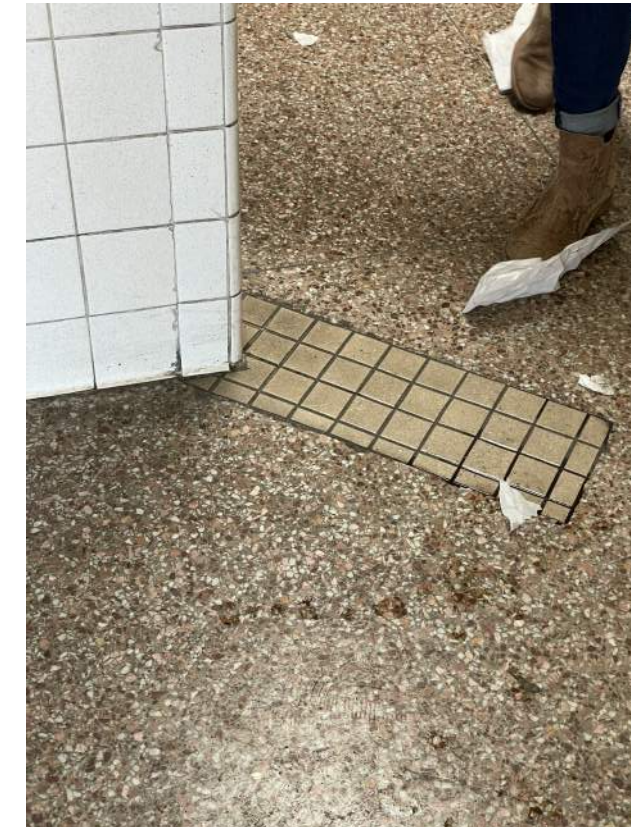
Image 2.3.3 Patched restroom floor. Taken on 04/27/2022 by Belli Architectural Group.
