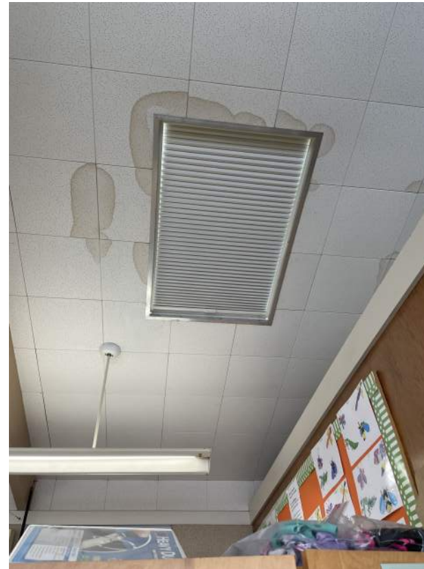
Image 2.3.1 Damaged ceiling panels. Taken on 04/27/2022 by Belli Architectural Group.
