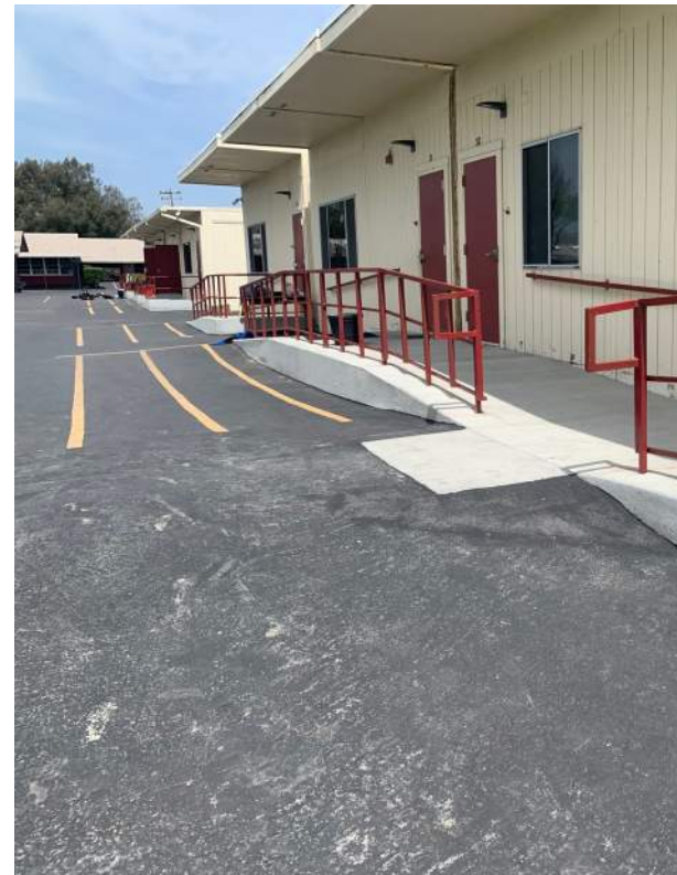
Image 2.1.2 Steep changes in asphalt elevation. Taken on 04/27/2022 by Belli Architectural Group.
