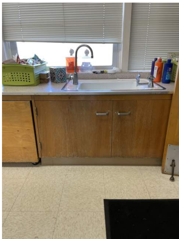
Image 2.3.3 Non-accessible sink at older casework. Taken on 05/03/2022 by Belli Architectural Group.
