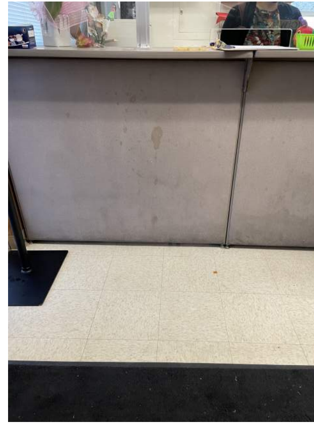
Image 2.3.1 Surface damage at reception desk. Taken on 05/03/2022 by Belli Architectural Group.
