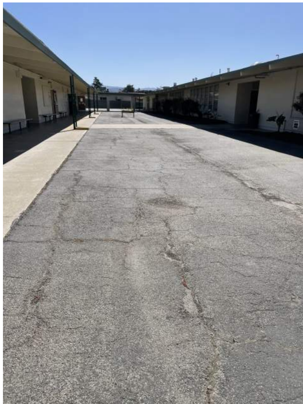
Image 2.1.1 Cracked, weathered conditions in asphalt. Taken on 05/03/2022 by Belli Architectural Group.
