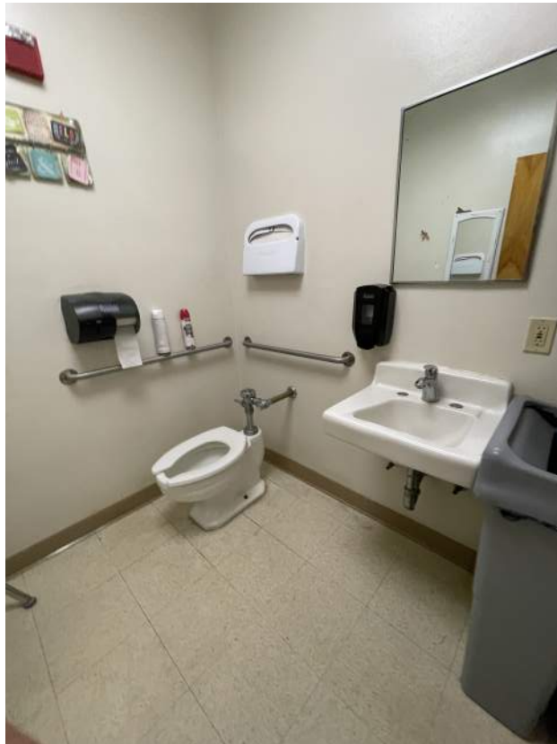
Image 2.4.1 Not fully ADA-compliant staff restroom. Taken on 05/03/2022 by Belli Architectural Group.
