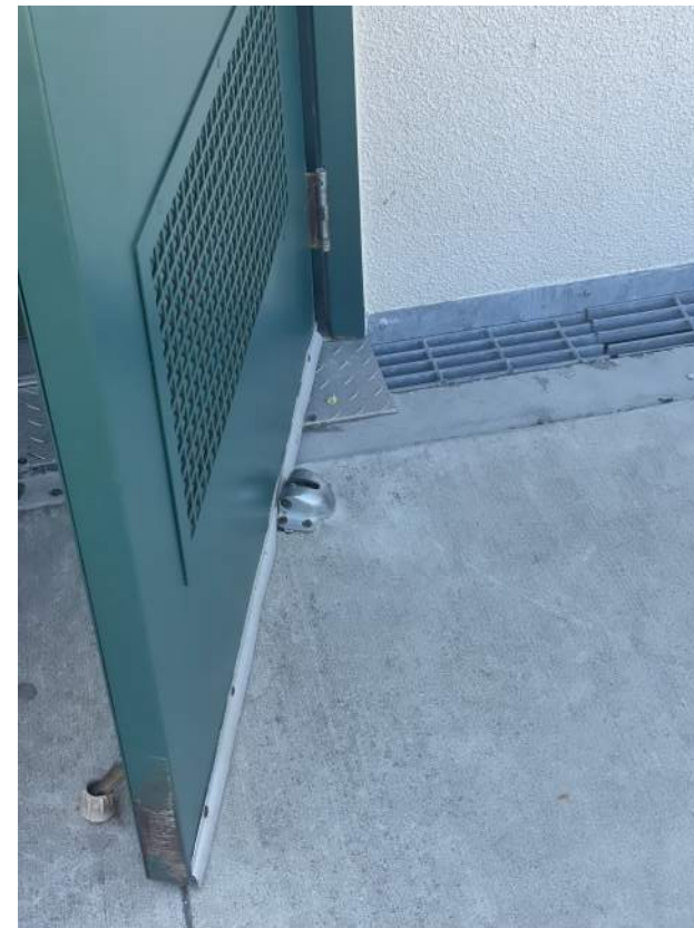
Image 2.4.2 Door stop at pit-set modular restroom. Taken on 05/03/2022 by Belli Architectural Group.
