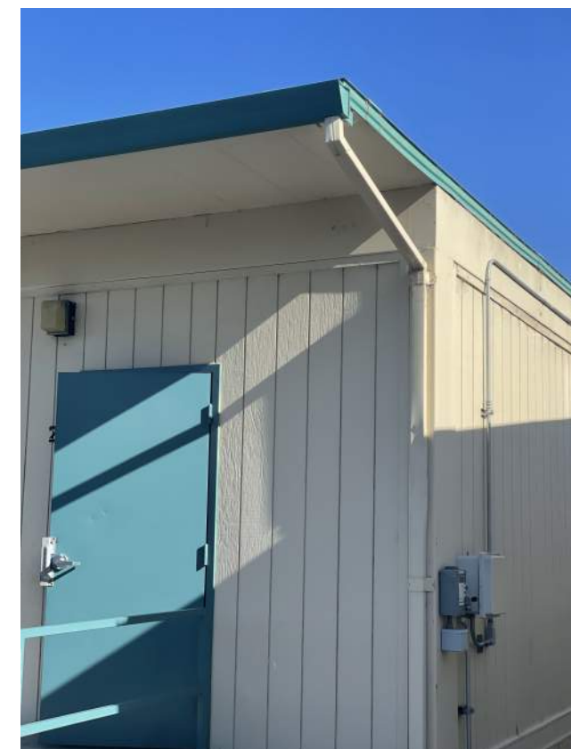
Image 2.2.5 Damaged gutter. Taken on 05/03/2022 by Belli Architectural Group.
