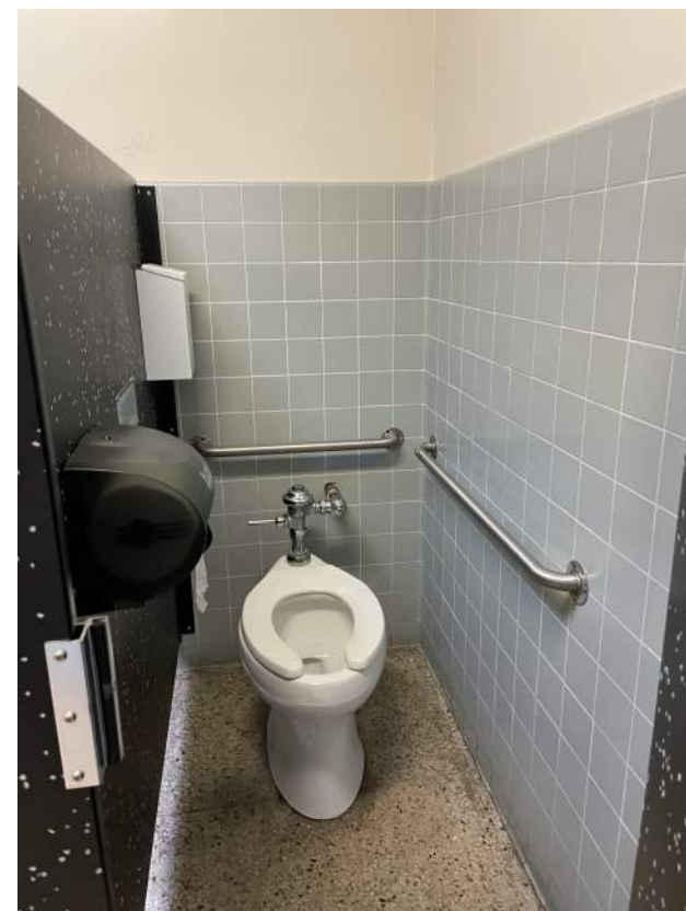
Image 2.4.3 Non-ADA compliant restroom. Taken on 05/03/2022 by Belli Architectural Group.
