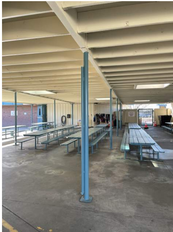
Image 2.1.1 Surfaces in need of seal coating. Taken on 05/03/2022 by Belli Architectural Group.
