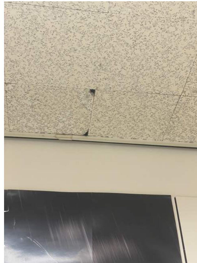
Image 2.3.2 Aging ceiling panels. Taken on 05/03/2022 by Belli Architectural Group.
