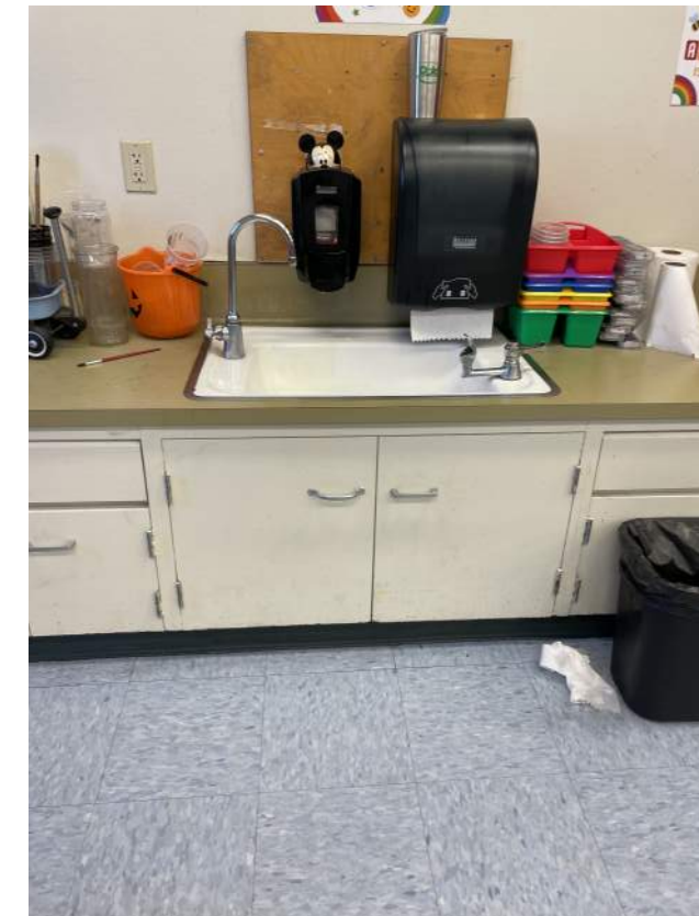
Image 2.4.4 Non-accessible sink. Taken on 05/03/2022 by Belli Architectural Group.
