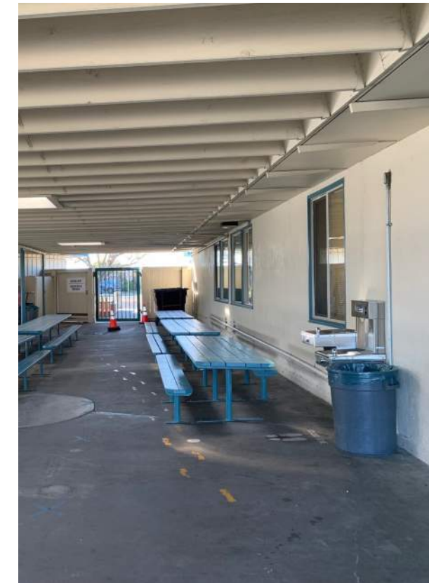
Image 2.1.4 Non-accessible drinking fountain. Taken on 05/03/2022 by Belli Architectural Group.
