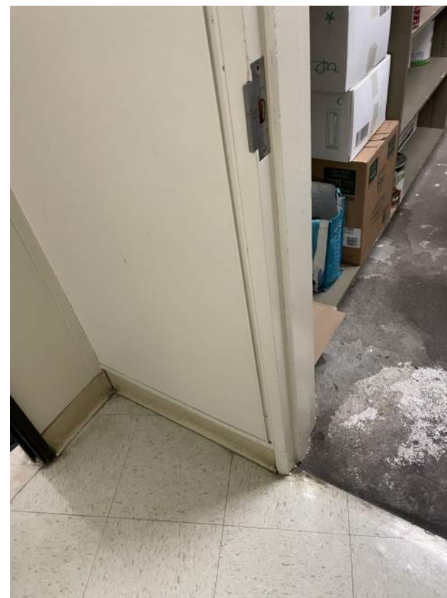
Image 2.3.3 Aging flooring. Taken on 05/03/2022 by Belli Architectural Group.
