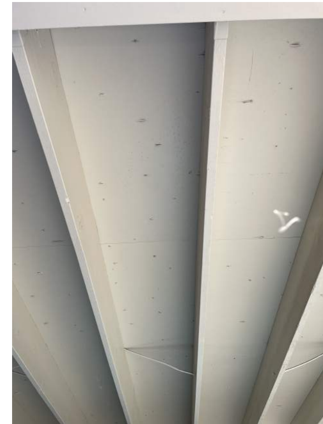
Image 2.2.4 Damaged plywood at fixed breezeway cover between MPR and Admin. Building. Taken on 05/03/2022 by Belli Architectural Group.
