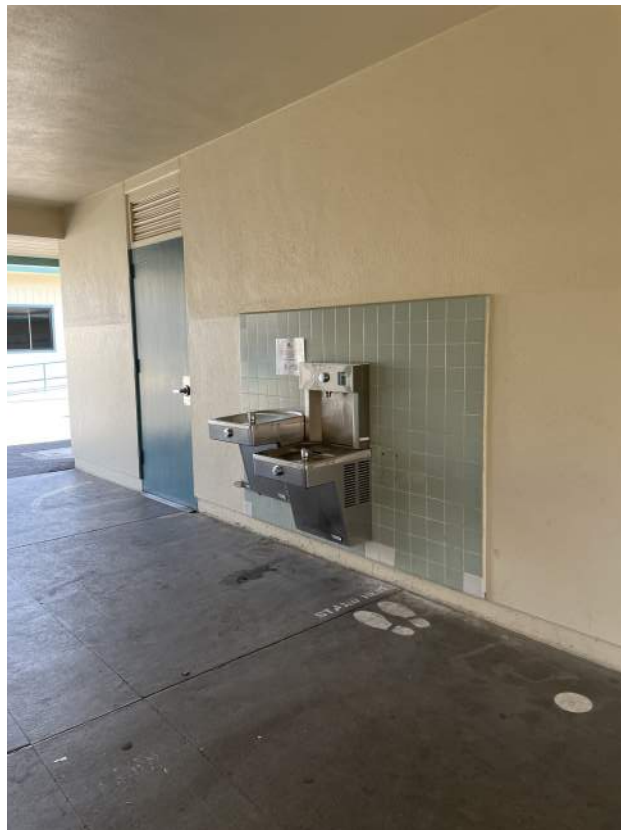
Image 2.4.1 Non-ADA compliant drinking fountain. Taken on 05/03/2022 by Belli Architectural Group.
