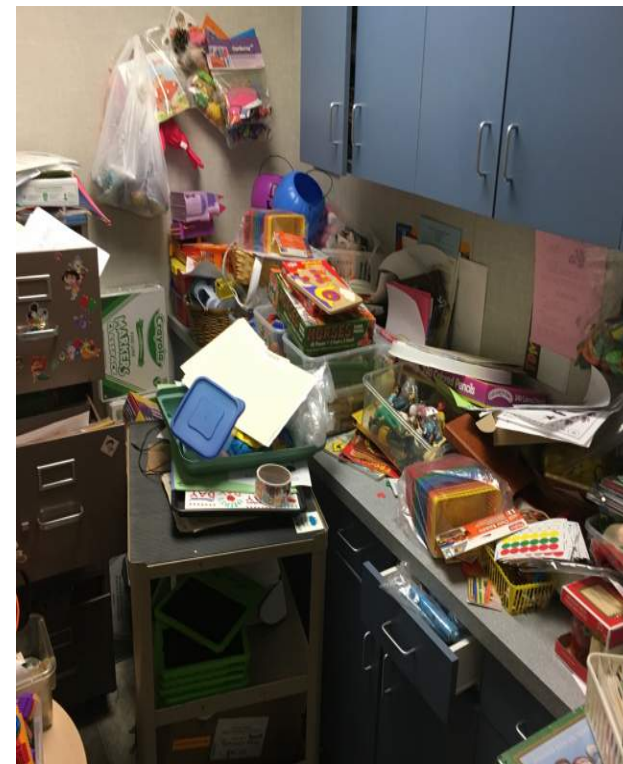
Image 2.3.9 Preschool. Small deteriorated spaces Taken on 05/03/2022 by Belli Architectural Group.
