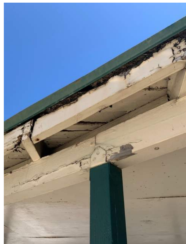
Image 2.2.6 Dry rot conditions at Library overhang. Taken on 05/03/2022 by Belli Architectural Group.
