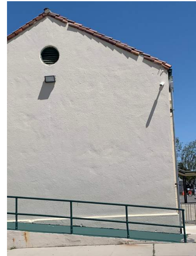
Image 2.2.7 Non-accessible ramp. Taken on 05/03/2022 by Belli Architectural Group.
