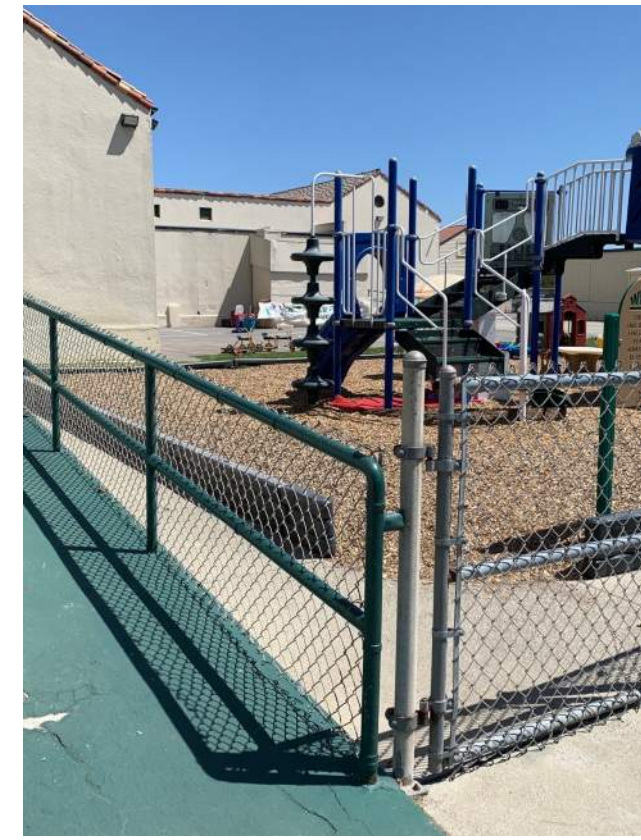
Image 2.1.5 Non-accessible ramp to kindergarten playground. Taken on 05/03/2022 by Belli Architectural Group.
