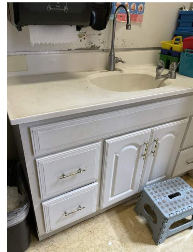
Image 2.3.10 Classroom casework. Taken on 05/03/2022 by Belli Architectural Group.
