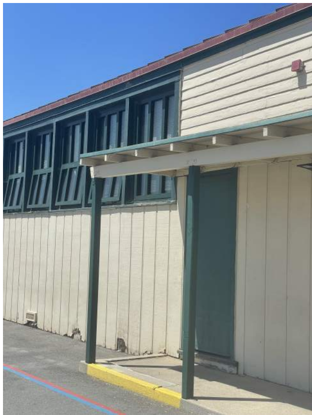
Image 2.2.10 Non-accessible door at relocatable classroom. Taken on 05/03/2022 by Belli Architectural Group.
