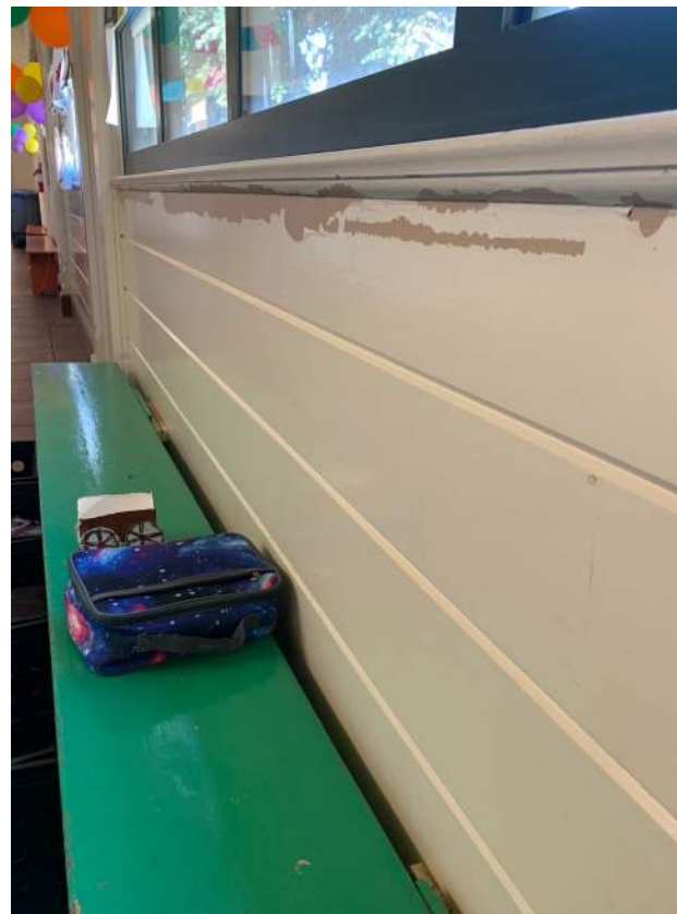
Image 2.3.2 Peeling interior paint. Taken on 05/03/2022 by Belli Architectural Group.
