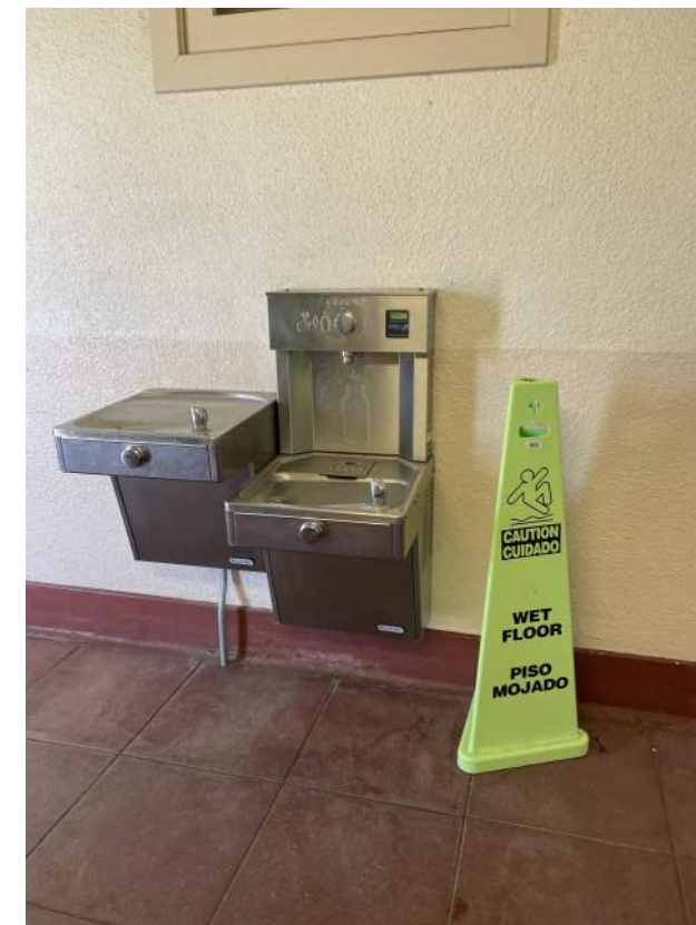
Image 2.4.2 Drinking fountain missing cane detection rails. Taken on 05/03/2022 by Belli Architectural Group.
