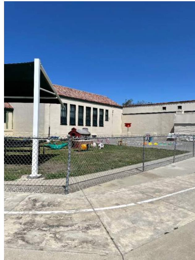
Image 2.1.7 Aging concrete surfaces. Taken on 05/03/2022 by Belli Architectural Group.
