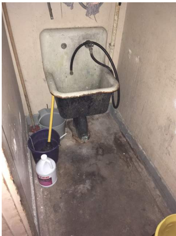
Image 2.3.12 Janitorial room. Taken on 05/03/2022 by Belli Architectural Group.
