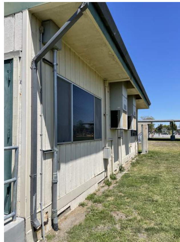
Image 2.2.12 Rusted HVAC units. Taken on 05/03/2022 by Belli Architectural Group.
