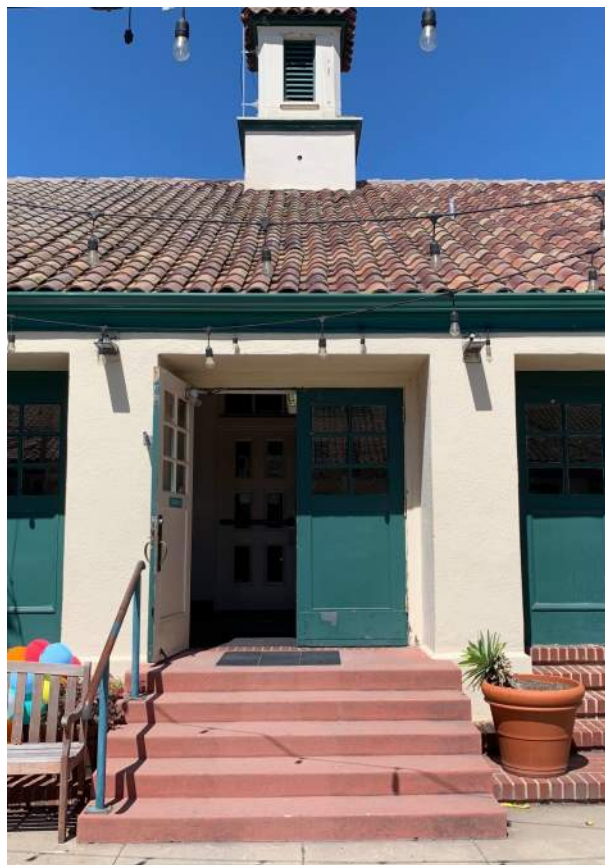
Image 2.1.6 Rusty handrail. Taken on 05/03/2022 by Belli Architectural Group.
