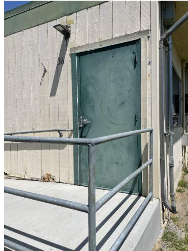
Image 2.2.11 Weathered exterior conditions and dry rot at portables. Taken on 05/03/2022 by Belli Architectural Group.
