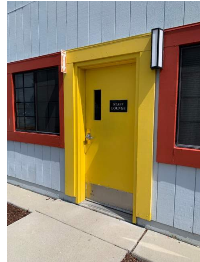
Image 2.2.5 Non-compliant door threshold. Taken on 04/26/2022 by Belli Architectural Group.
