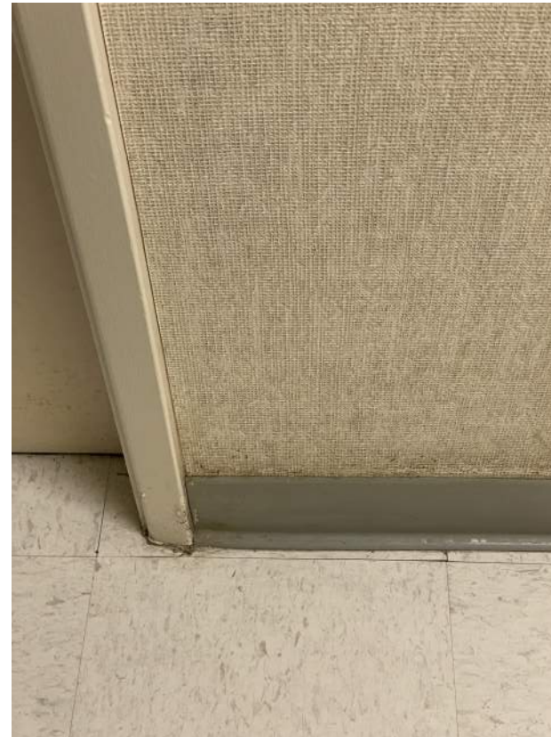
Image 2.3.2 Worn, dirty walls and floor finishes. Taken on 04/26/2022 by Belli Architectural Group.
