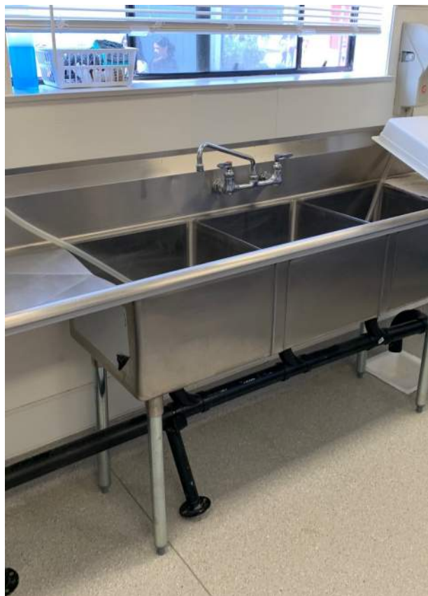
Image 2.3.7 Sink at MPR does not drain properly. Taken on 04/26/2022 by Belli Architectural Group.
