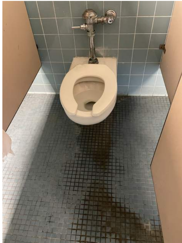
Image 2.3.6 Plumbing leak. Taken on 04/26/2022 by Belli Architectural Group.
