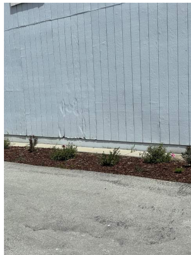
Image 2.2.5 Dry rot present at exterior wood paneling. Taken on 04/26/2022 by Belli Architectural Group.
