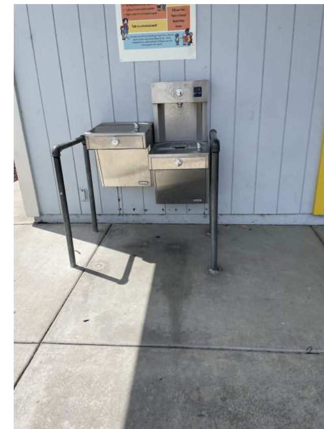
Image 2.4.3 Non-accessible drinking fountain. Taken on 04/26/2022 by Belli Architectural Group.
