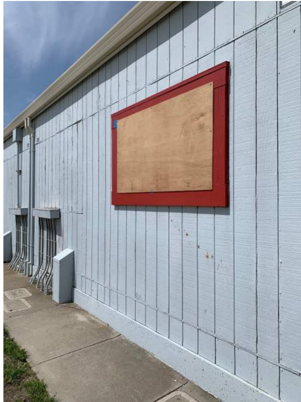
Image 2.2.2 Missing window. Taken on 04/26/2022 by Belli Architectural Group.
