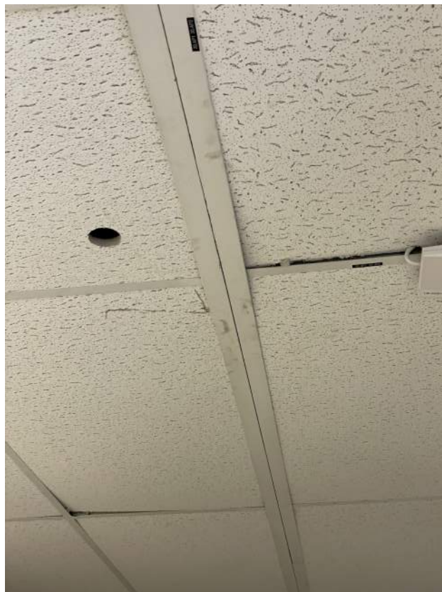
Image 2.3.1 Damaged ceiling panels. Taken on 04/26/2022 by Belli Architectural Group.
