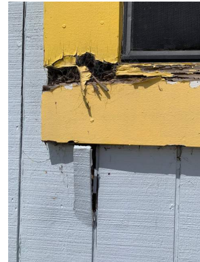
Image 2.2.1 Exterior dry rot. Taken on 04/26/2022 by Belli Architectural Group.
