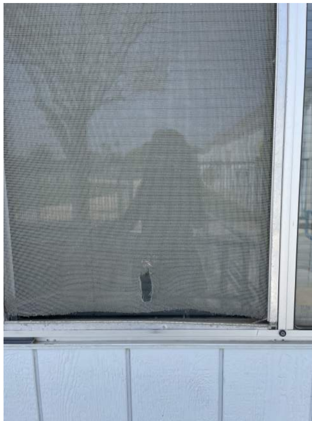
Image 2.2.3 Broken screens. Taken on 04/26/2022 by Belli Architectural Group.
