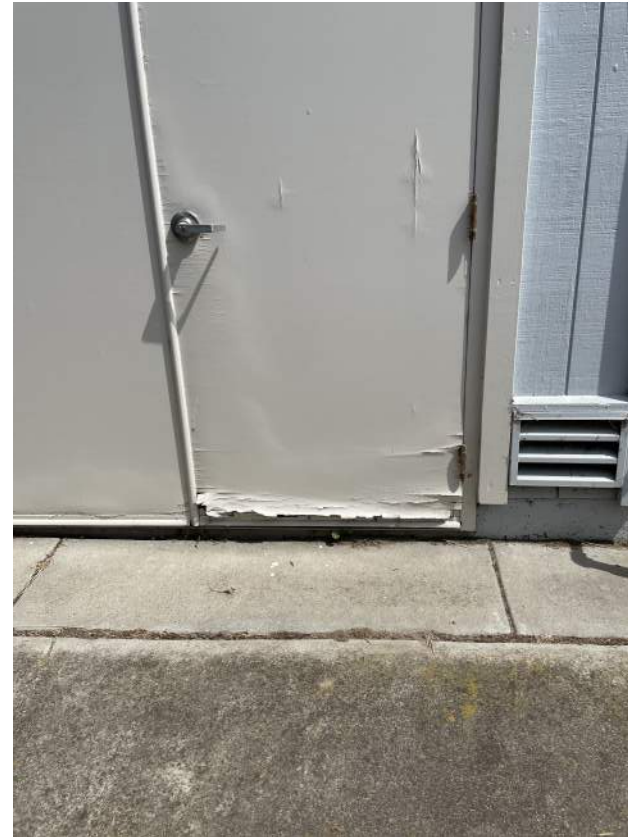
Image 2.2.4 Dry rot present at most exterior doors. Taken on 04/26/2022 by Belli Architectural Group.
