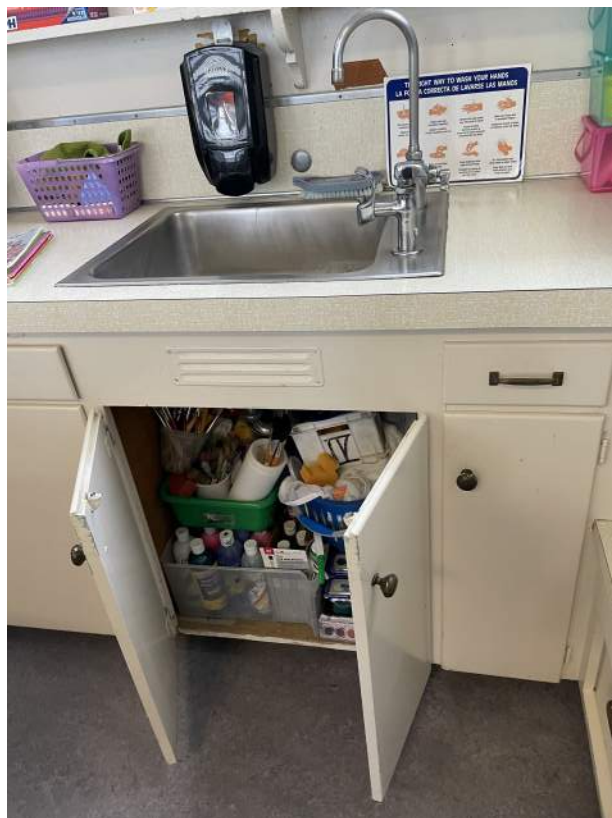
Image 2.2.10 Classroom casework. Taken on 04/26/2022 by Belli Architectural Group.
