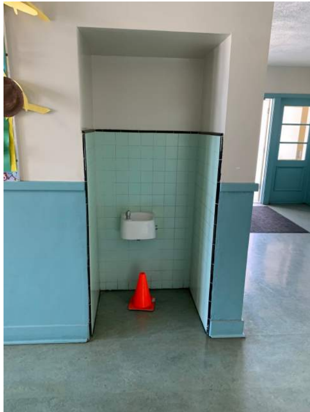
Image 2.4.3 Non-accessible drinking fountain. Taken on 04/26/2022 by Belli Architectural
