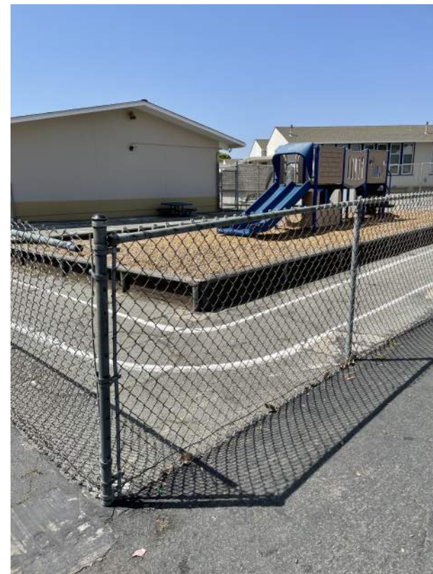
Image 2.1.3 Non-accessible deteriorated Kindergarten playground. Taken on 04/26/2022 by Belli Architectural Group.
