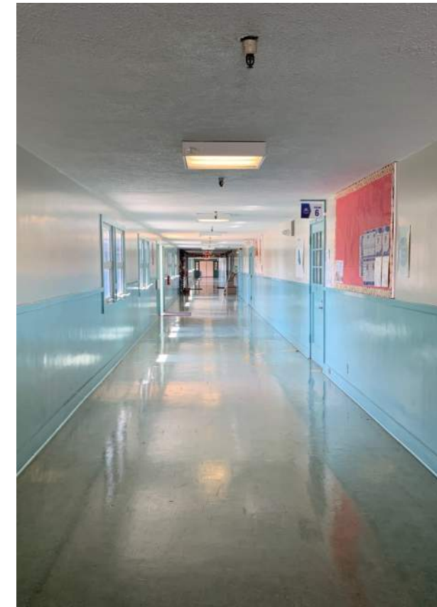
Image 2.2.7 Aging hallway flooring. Taken on 04/26/2022 by Belli Architectural Group.
