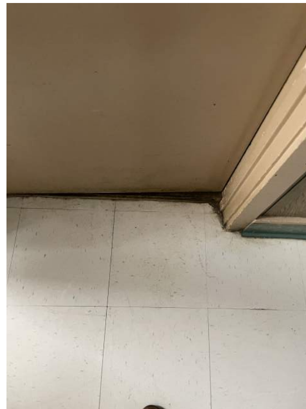
Image 2.2.5 Dirt accumulated at floors and walls. Taken on 04/26/2022 by Belli Architectural Group.
