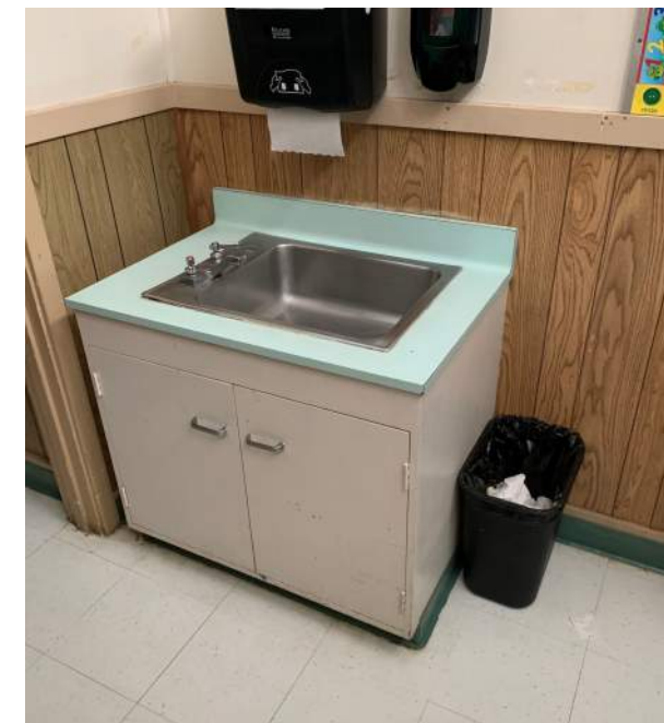
Image 2.4.2 Non-accessible sink at classroom. Taken on 04/26/2022 by Belli Architectural Group.
