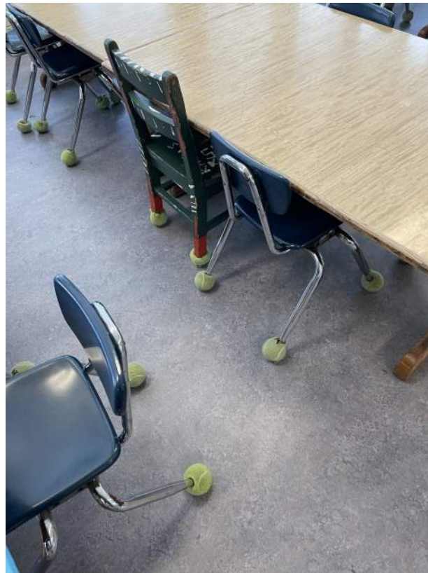
Image 2.2.9 Existing chairs damage floor surface. Taken on 04/26/2022 by Belli Architectural Group.
