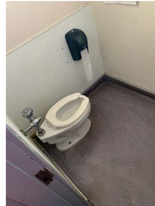
Image 2.4.1 Non-accessible restrooms. Taken on 04/26/2022 by Belli Architectural Group.
