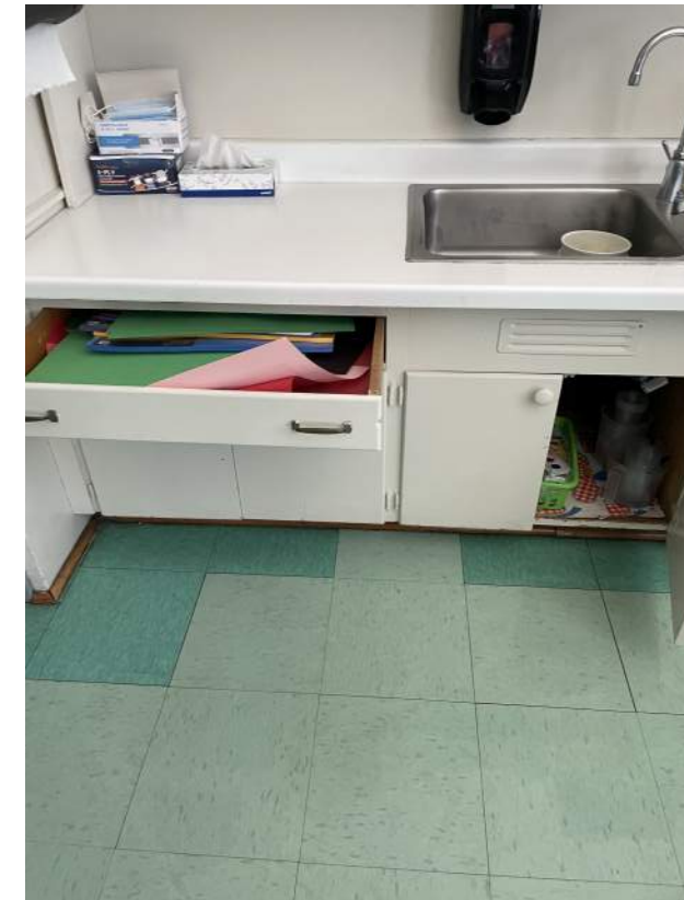
Image 2.3.1 Older, patched flooring at non-accessible classroom sink. Taken on 04/26/2022 by Belli Architectural Group.
