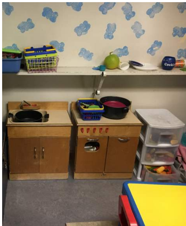
Image 2.3.16 Preschool. Non-accessible sink. Taken on 04/26/2022 by Belli Architectural Group.
