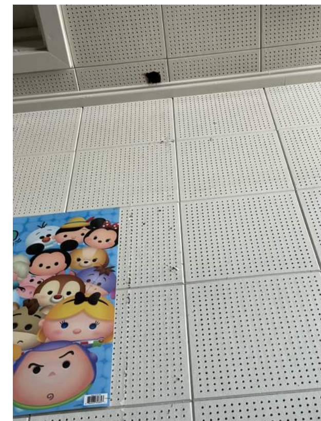
Image 2.3.2 Broken and aging acoustic panels. Taken on 04/26/2022 by Belli Architectural Group.
