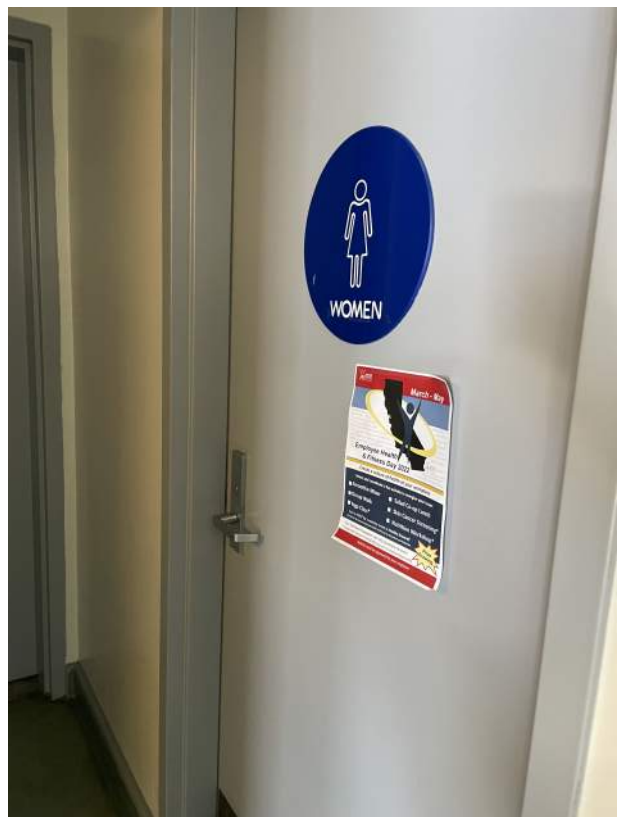
Image 2.4.4 Missing restroom wall signage. Taken on 04/26/2022 by Belli Architectural Group.
