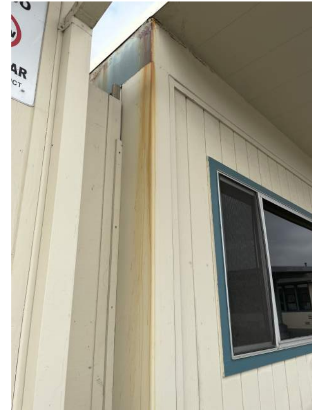
Image 2.2.7 Rust present at relocatable classrooms. Taken on 05/02/2022 by Belli Architectural Group.
