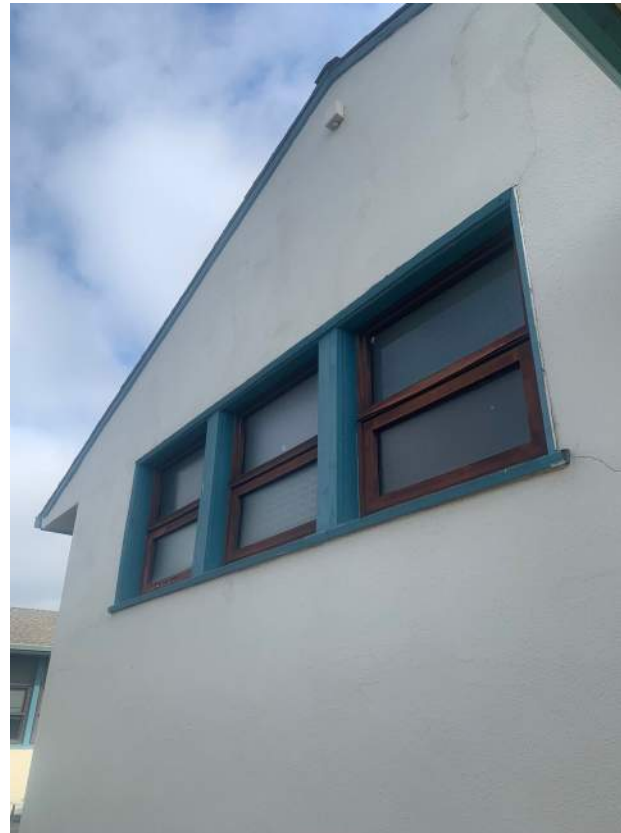
Image 2.2.5 Plaster cracks. Taken on 05/02/2022 by Belli Architectural Group.
