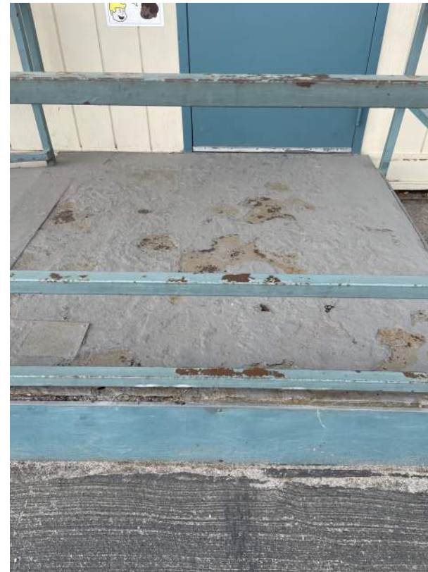
Image 2.1.1 Rot and rust at portable classroom ramps. Taken on 05/02/2022 by Belli Architectural Group.
