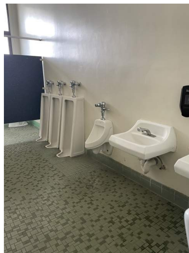
Image 2.3.8 Missing privacy partitions between urinals and sinks. Taken on 05/02/2022 by Belli Architectural Group.
