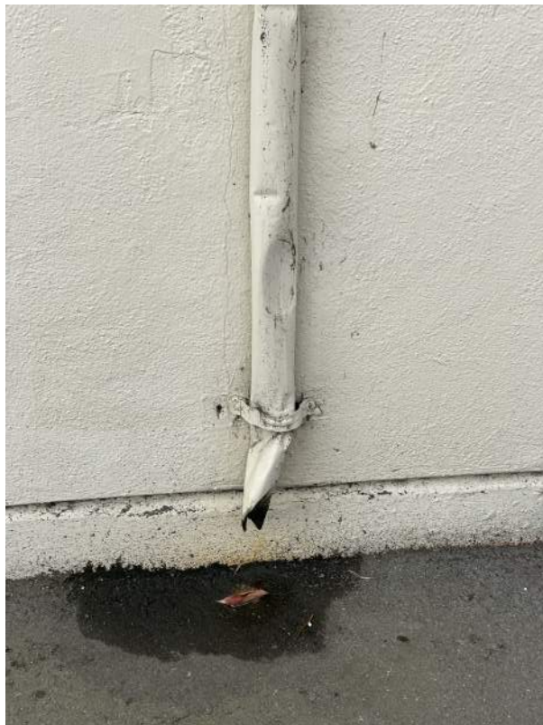
Image 2.2.4 Damaged gutter. Taken on 05/02/2022 by Belli Architectural Group.
