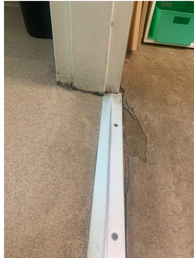
Image 2.3.7 Damaged flooring. Taken on 05/02/2022 by Belli Architectural Group.
