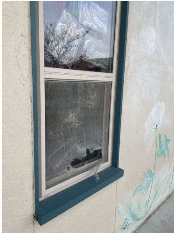
Image 2.2.3 Broken window screens. Taken on 05/02/2022 by Belli Architectural Group.
