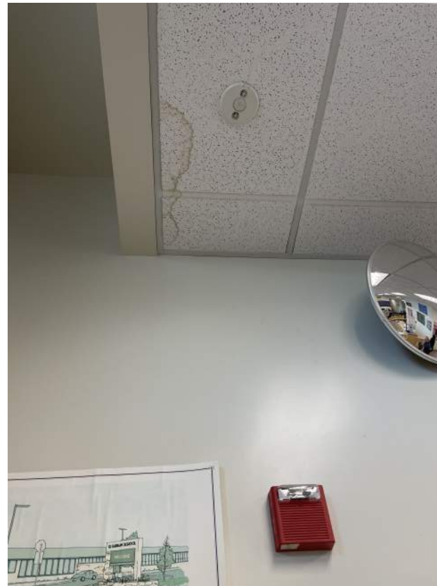
Image 2.3.1 Damaged ceiling panel. Taken on 05/02/2022 by Belli Architectural Group.
