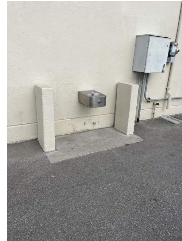
Image 2.1.3 Non-ADA compliant drinking fountain. Taken on 05/02/2022 by Belli Architectural Group.
