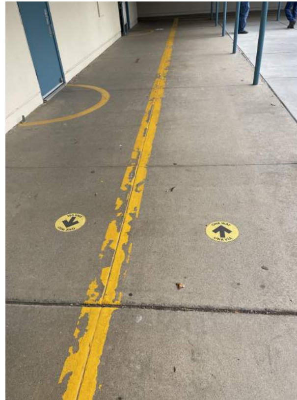
Image 2.1.1 Worn off exterior pavement striping. Taken on 05/02/2022 by Belli Architectural Group.
