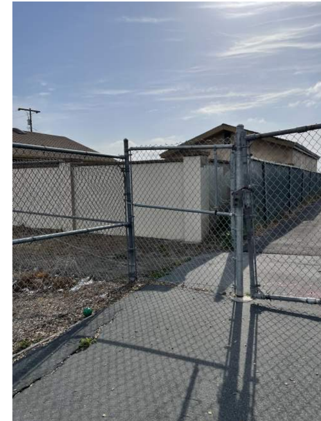
Image 2.1.5 Damaged fence. Taken on 04/26/2022 by Belli Architectural Group.
