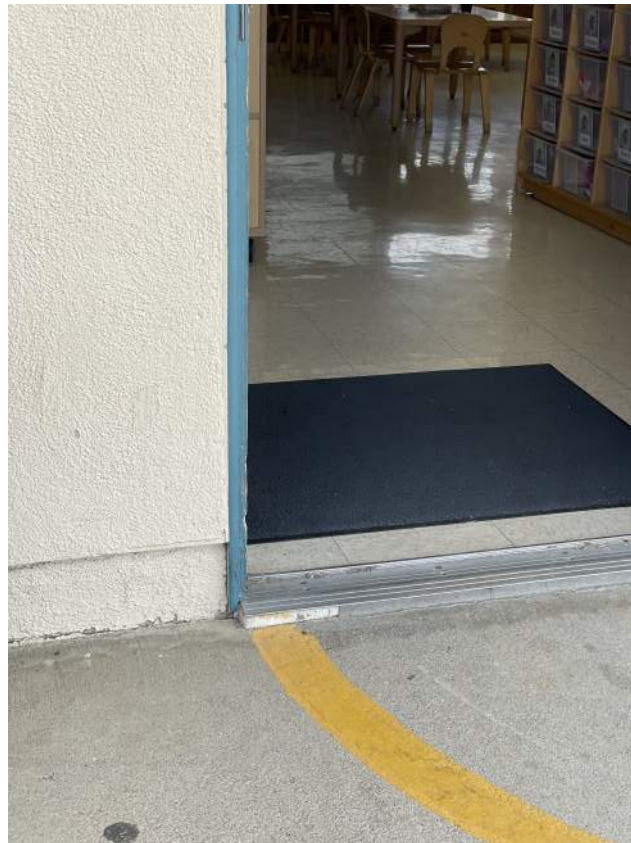
Image 2.2.3 Non-ADA compliant threshold. Taken on 04/26/2022 by Belli Architectural Group.
