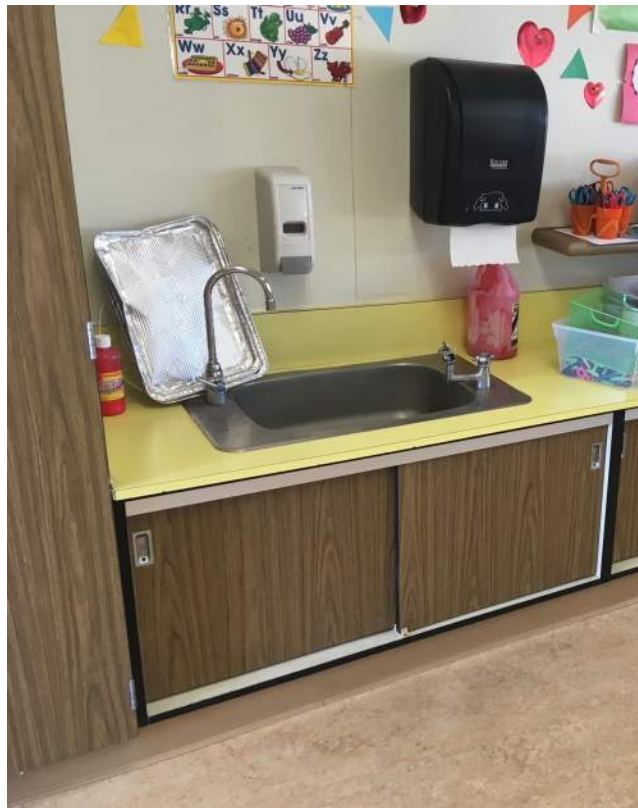
Image 2.3.13 Preschool. Non-compliant sink. Taken on 04/26/2022 by Belli Architectural Group.
