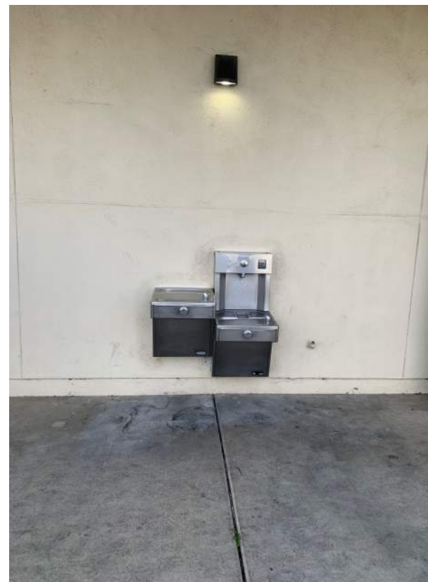
Image 2.4.2 Drinking fountains missing cane rails detection. Taken on 04/26/2022 by Belli Architectural Group.
