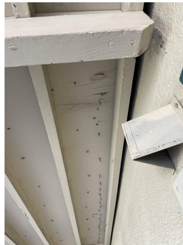
Image 2.2.6 Exposed nails present at portable classrooms. Taken on 04/26/2022 by Belli Architectural Group.
