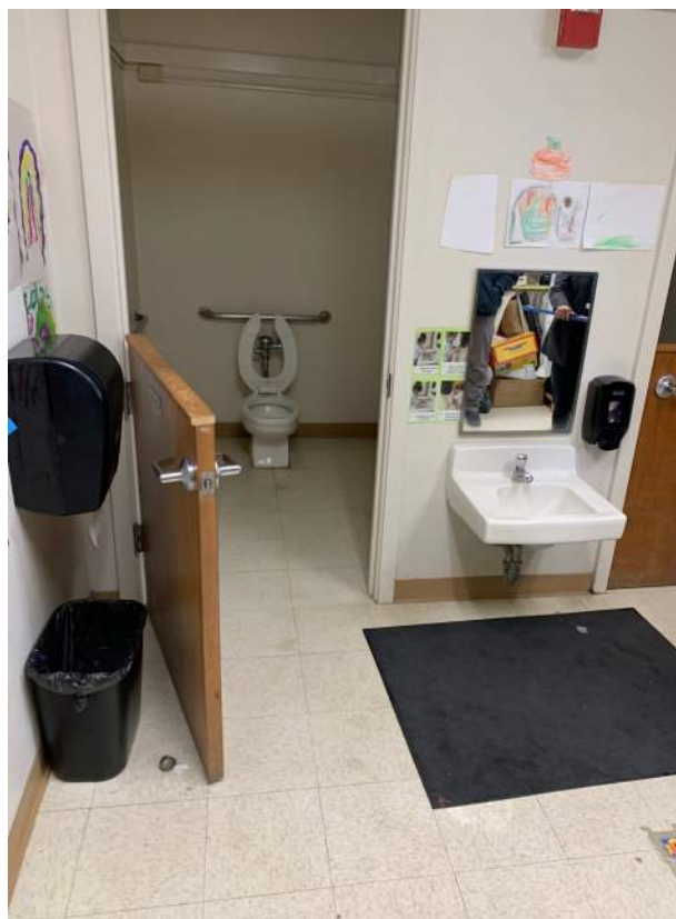
Image 2.3.8 Existing non-compliant Kindergarten restrooms. Taken on 04/26/2022 by Belli Architectural Group.
