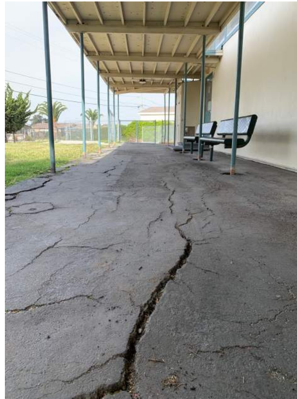
Images 2.1.2 Damaged walkways. Taken on 04/26/2022 by Belli Architectural Group.
