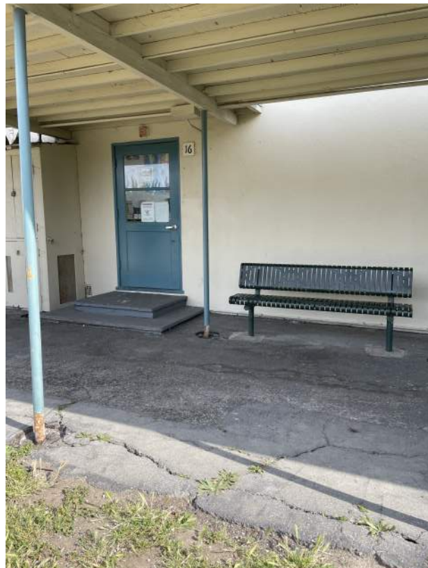
Image 2.1.1 Damaged walkways. Taken on 04/26/2022 by Belli Architectural Group.
