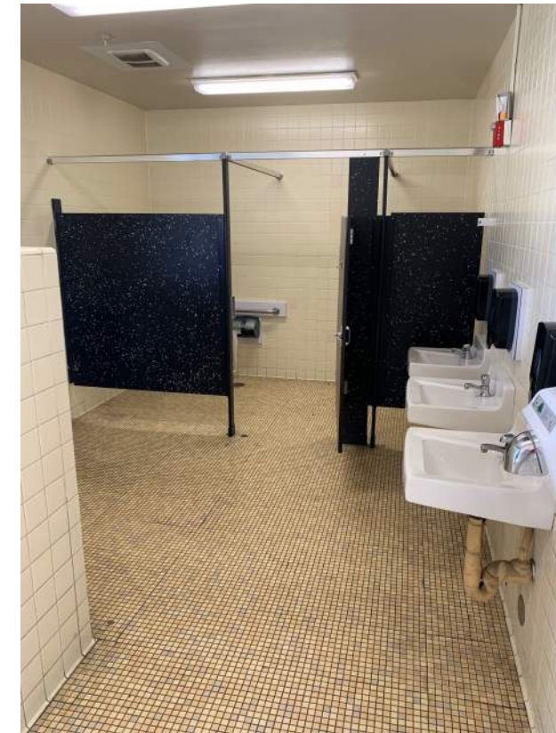
Image 2.3.11 Outdated, worn restroom conditions. Taken on 04/26/2022 by Belli Architectural Group.
