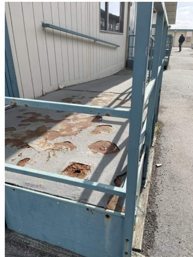
Image 2.2.5 Rust and holes present at portable access ramps. Taken on 04/26/2022 by Belli Architectural Group.
