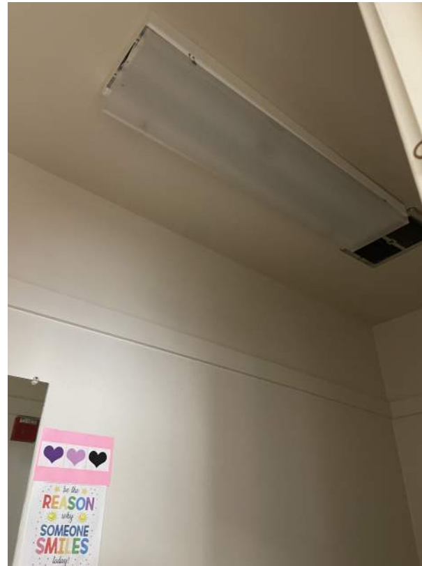
Image 2.3.1 Damaged light fixture. Taken on 04/26/2022 by Belli Architectural Group.
