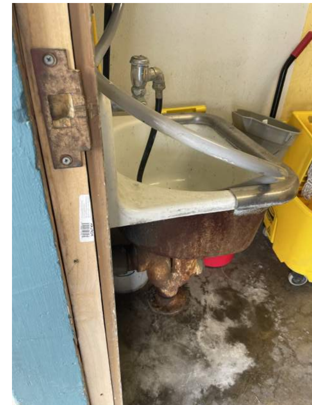
Image 2.3.6 Rust and deterioration at Janitorial Room. Taken on 04/26/2022 by Belli Architectural Group.
