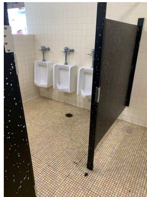
Image 2.3.10 Outdated, worn restroom conditions. Taken on 04/26/2022 by Belli Architectural Group.
