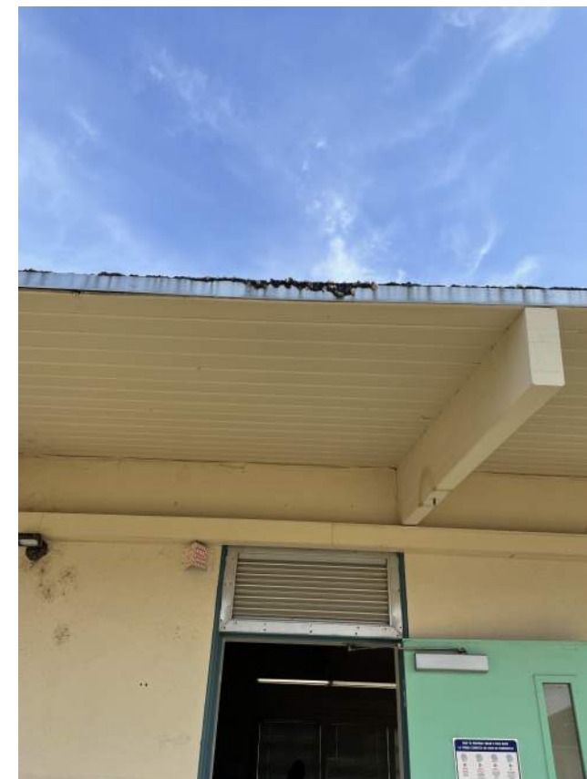
Image 2.2.2 Failing conditions at existing roof. Taken on 04/26/2022 by Belli Architectural Group.
