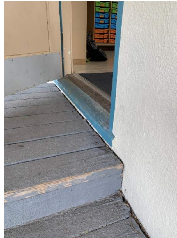
Image 2.4.1 Non-accessible entrance to classrooms. Taken on 04/26/2022 by Belli Architectural Group.
