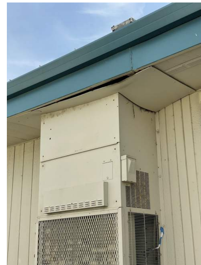
Image 2.2.8 Collapsing soffit at portable classroom. Taken on 04/26/2022 by Belli Architectural Group.
