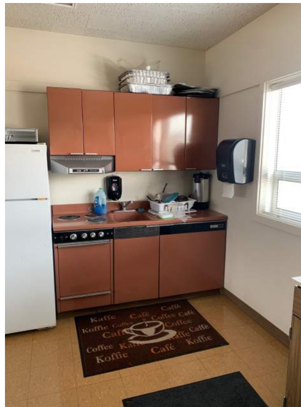
Image 2.3.3 Non-accessible sink at Staff Lounge. Taken on 04/26/2022 by Belli Architectural Group.
