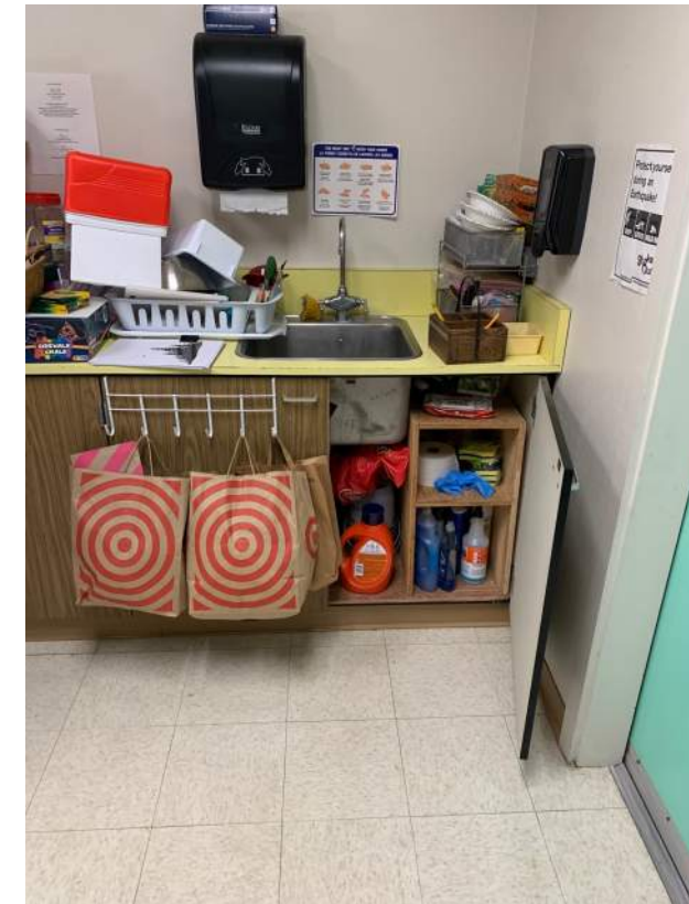
Image 2.3.5 Older finish materials and non-accessible sink. Taken on 04/26/2022 by Belli Architectural Group.
