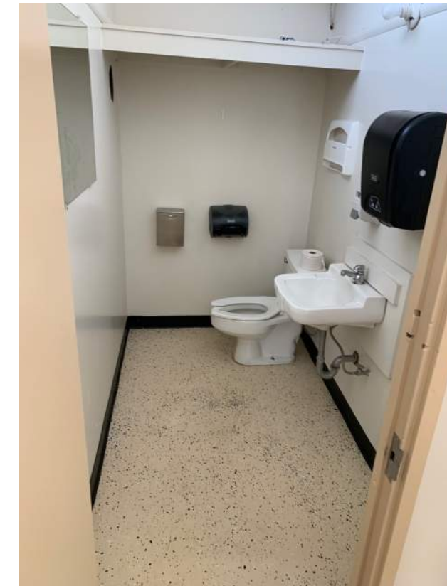
Image 2.4.3 Non-ADA compliant staff restrooms. Taken on 04/26/2022 by Belli Architectural Group.
