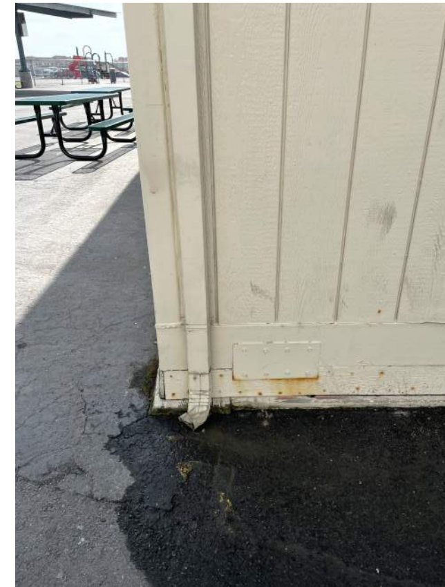
Image 2.2.7 Damaged gutter at portable classroom. Taken on 04/26/2022 by Belli Architectural Group.
