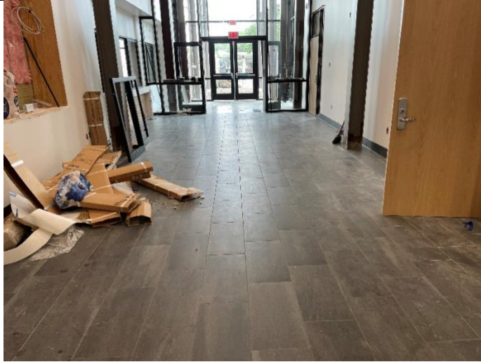
Area A: View of porcelain tile installation in Area A, Main entrance.
