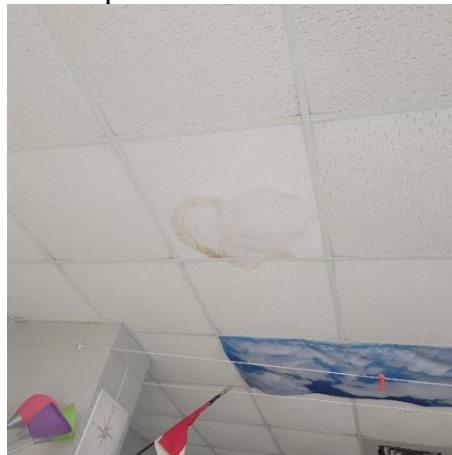
Representative staining on an acoustic ceiling tile
