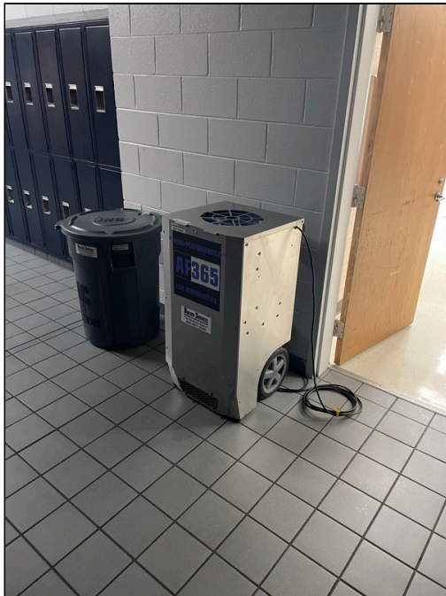
4 - Dehumidifiers were noted to be operating throughout each facility
