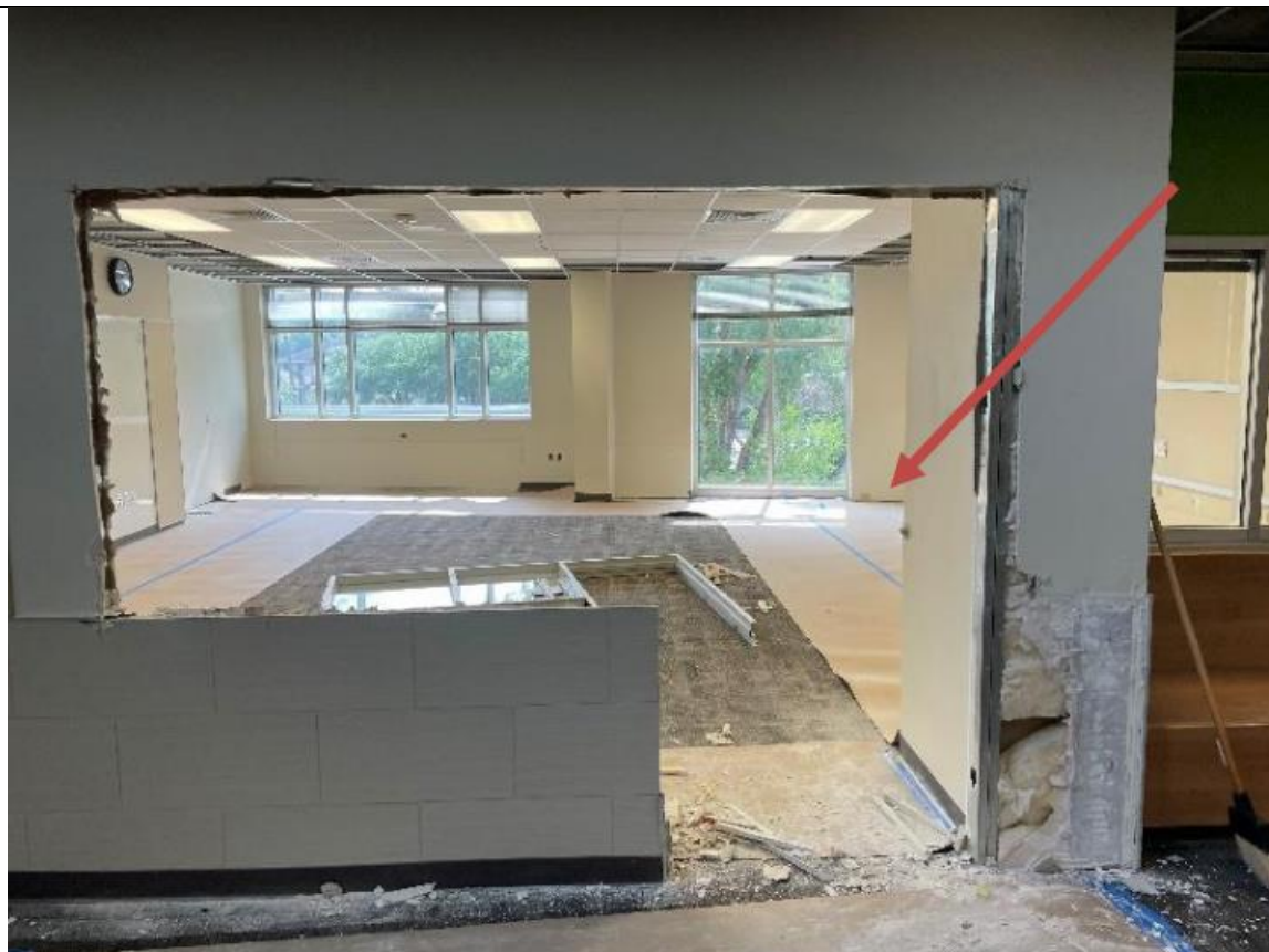
Interior demolition at existing classrooms for temporary construction barriers to go up.
