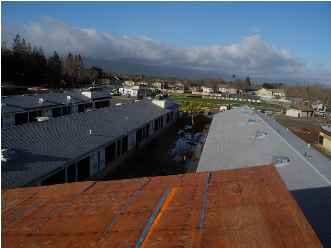
Roofs of school wings A, B and D at Steindorf from the top of the Admin. Building (wing C)
