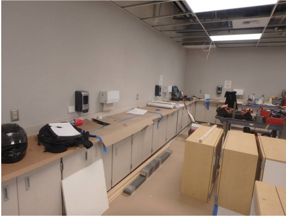
Alt. 1 main room looking south along the east wall and staged casework
