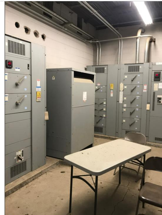
Main Electrical Room
