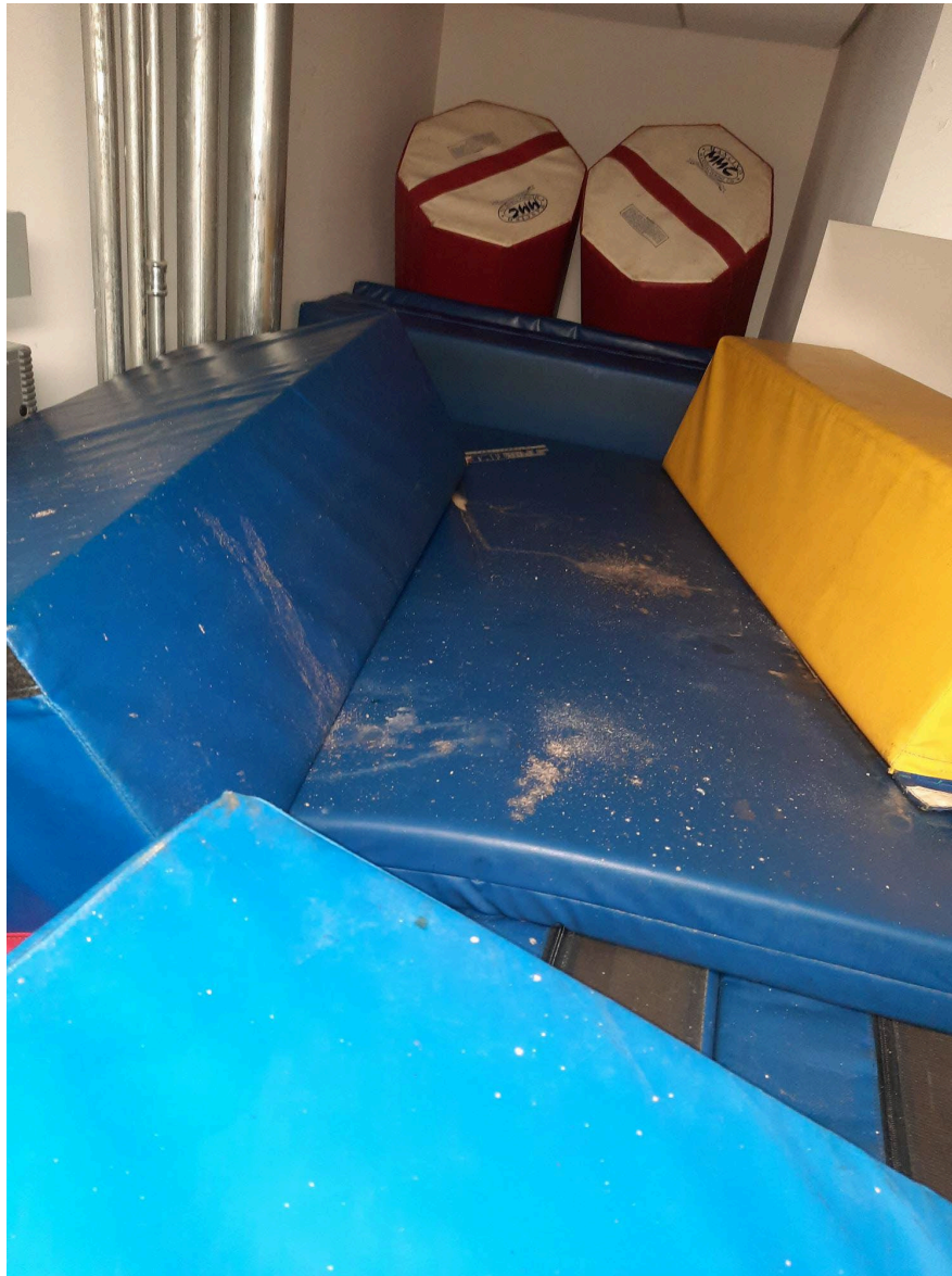
Physical Education Storage Room : Debris from water damaged ceiling tiles ( previously removed) was observed on mats.
