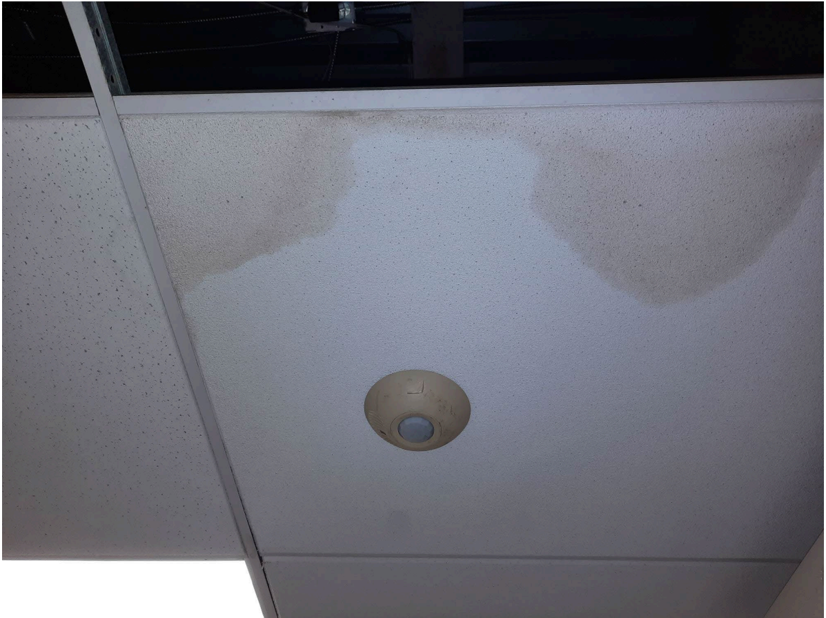
Physical Education Office : ~2 SF of water damaged ceiling tile
