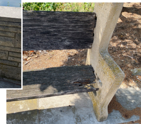
The wood on the benches needs replacement.
